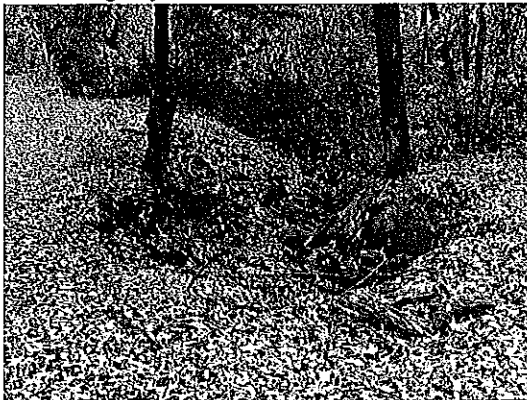
Photo: Existing stormwater runoff has created severe gully erosion along portions of Pheasant Branch Creek.
