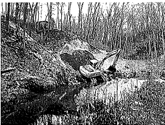
Photo: Topsoil being applied to the newly graded slope as part of the additional rootwad installations completed in November 2008.
