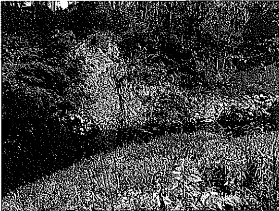
Photo: New rootwad revetment site located upstream from existing treatment prior to construction (note upstream end of stone treatment)
