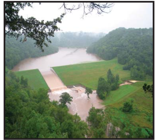
Floodwaters flowing over the emergency concrete spillway of the Springville Dam on the Springville Branch of the Bad Axe River. August 20, 2007.
