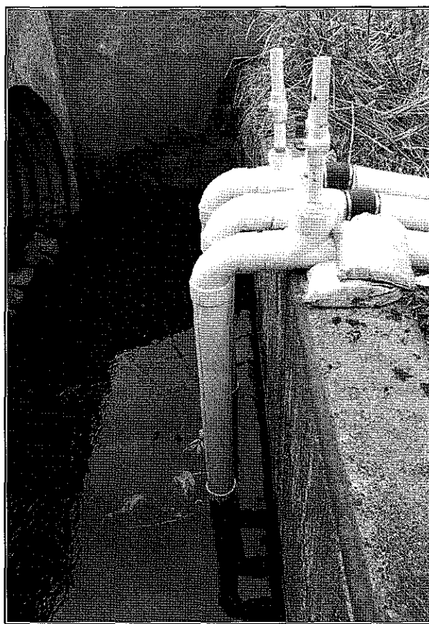
Figure 2. Siphons are constructed using 6" PVC pipe and fittings.
