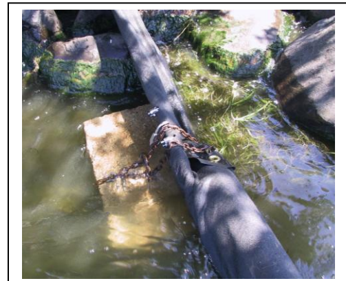
Fig. 5. Concrete block and chain used to prevent boom wall from being lifted out of lake at shoreline. (Photo: R. Lathrop, WDNR)
