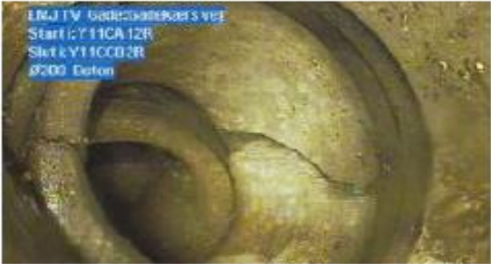
Cracked Sewer Pipe (Riis)
