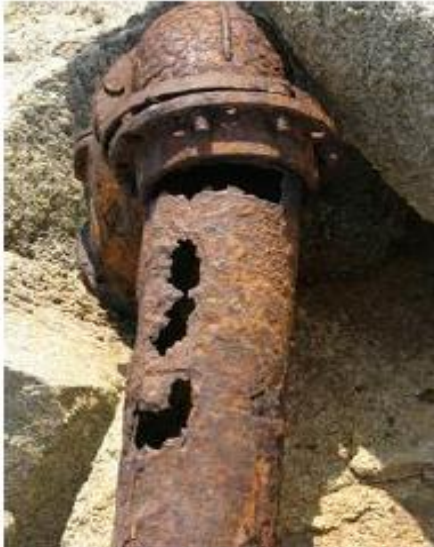
Corroded Sewer Pipe
