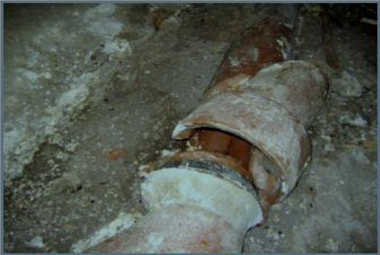
Separated Sewer Pipe
