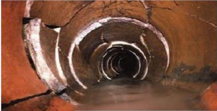
Cracked Sewer Pipes
