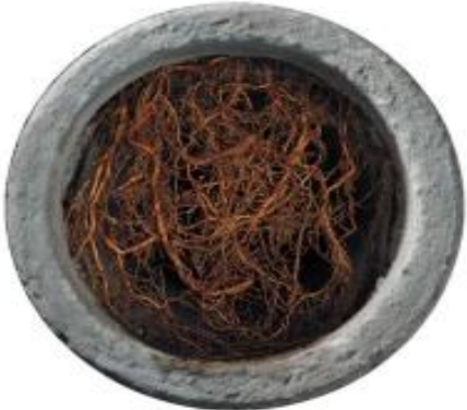
Rootlets in Sewer
