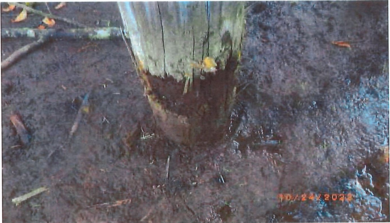
CS3 Timber pile decay. Measurable section loss.
