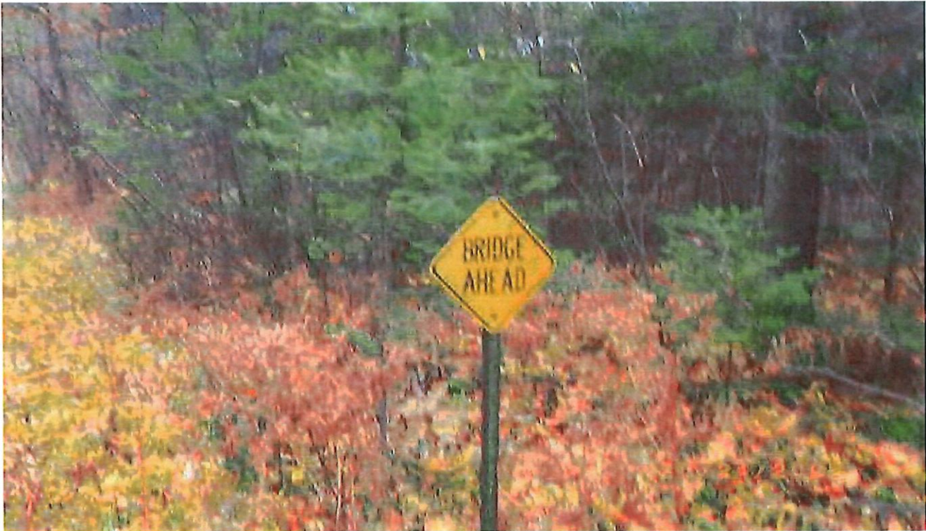
West Bridge Ahead sign, CS3 map cracked and no reflectivity.
