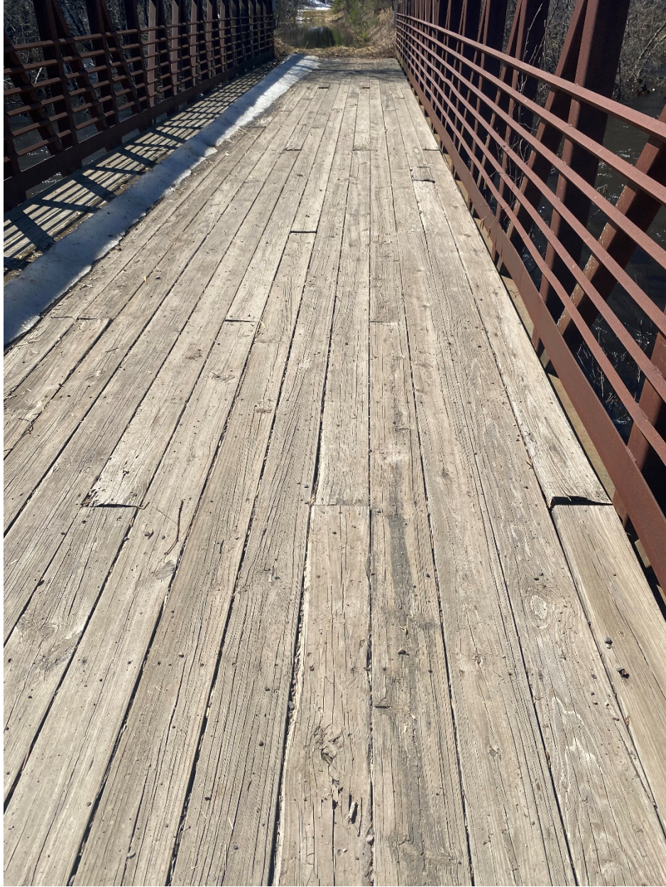
Looking west at the damaged bridge decking.
