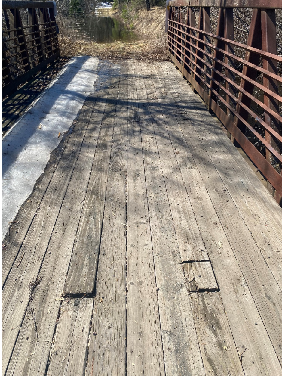
Looking west from bridge center at the damaged bridge decking.
