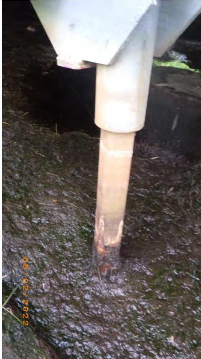
B1, Typical Helical, corrosion.
