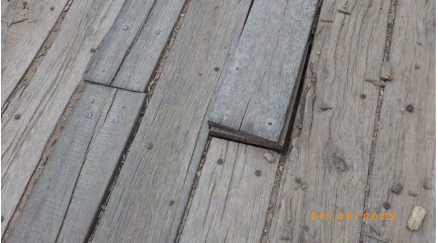
B1- CS3 loose deck boards.
