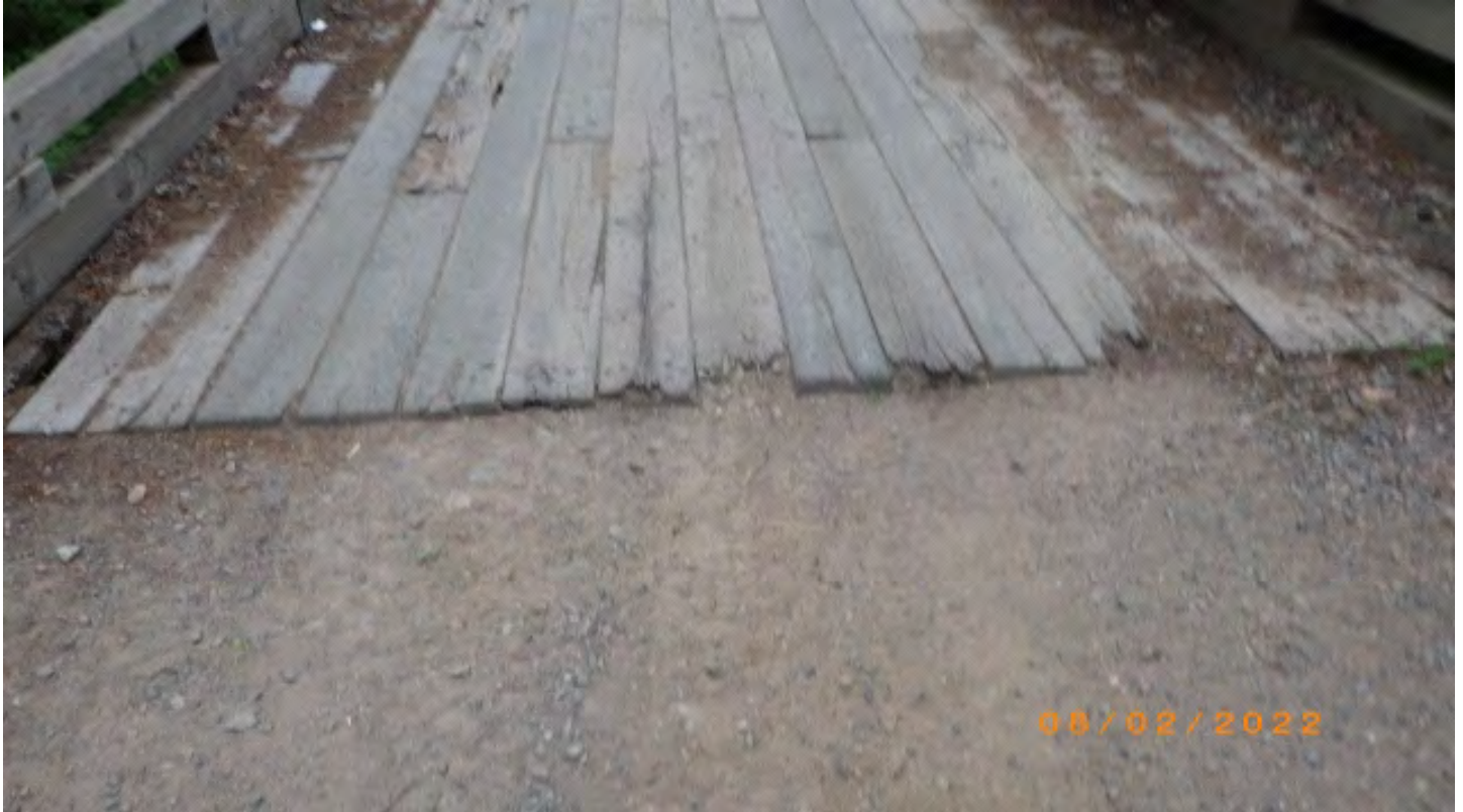
B3- 2inch settlement and CS3 deck boards.
