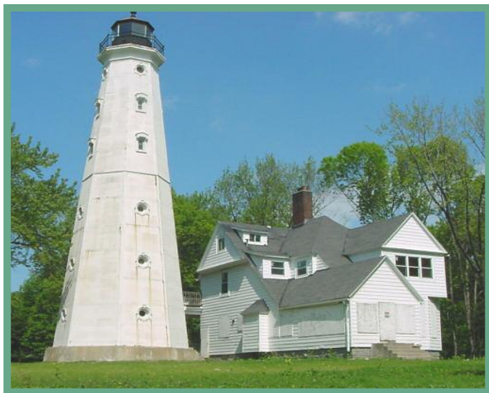
The North Point Lighthouse at Lake Park, prior to restoration work (photo courtesy DNR).
