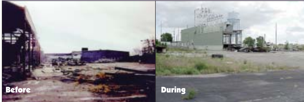
Left: The Radford Company site was a serious blight in the city of Oshkosh. (Photo courtesy of STS Consultants, Inc.) Right: Demolition of the Universal Foundry Building, another local eyesore, took place in 2000. (Photo courtesy of STS Consultants, Inc.)
