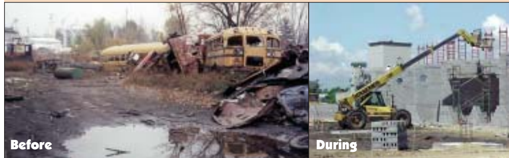
Left: The site of the new Baraboo City Services Center had many past uses, such as the scrapyard shown here, which contaminated the site (photo courtesy of MSA Professionals). Right: Construction of the new City Services Center began in 2001 (photo by Jessica Milz, DNR).
