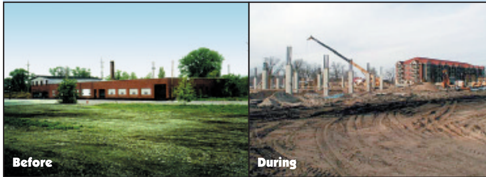
The CenturyTel, Inc., property before redevelopment [left] and after the beginning of construction of their new building in 1999 [right] (photos by Loren Brumberg and Dave Carper, DNR)
