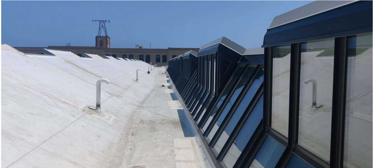
Picture 3 – Exhaust Fan Outlets on Building 4
