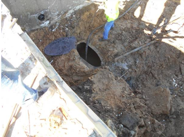
Photo #13 View looking north west at east tank during liquid removal/cleaning prior to removal.
