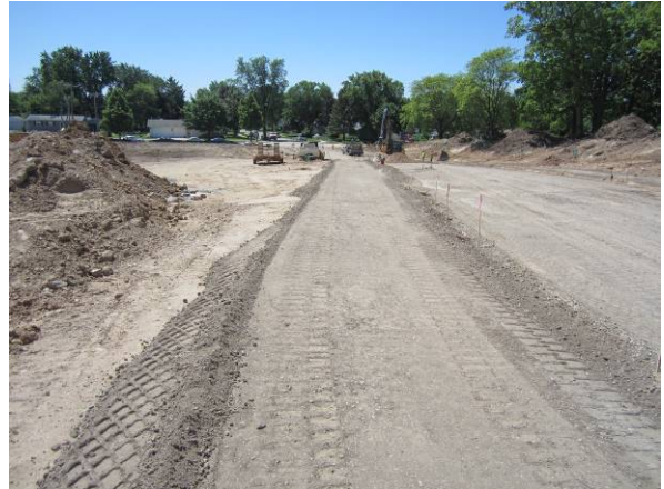
Photo #20 View looking south from Elliot Lane during construction of Elliot Lane
