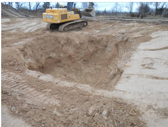
Photo #5 View of "vault area" where soil excavated from B-5/B-5A area was placed.
