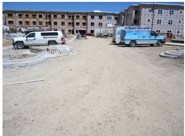
Photo #24 View looking north from central portion of site showing redevelopment activities.
