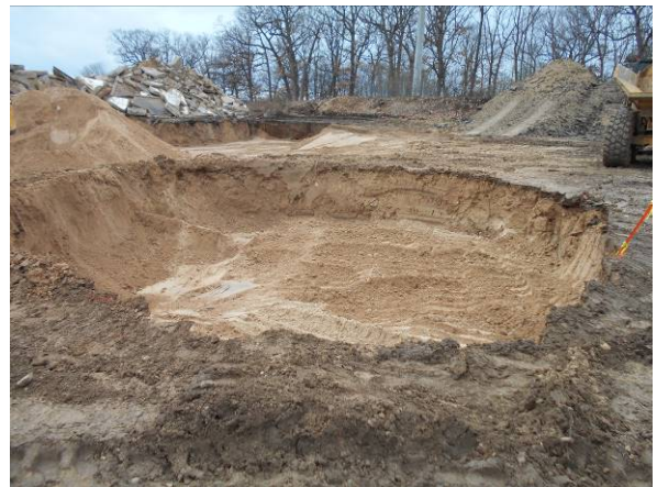
Photo #4 View looking south at B-5/B-5A excavation area after excavation was completed.
