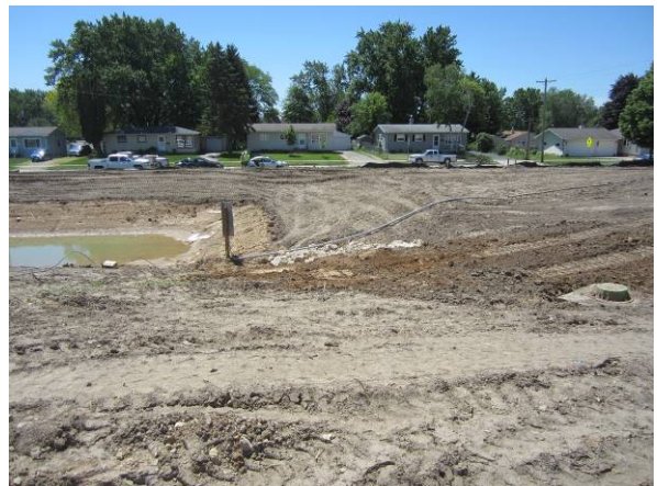
Photo #22 View looking south towards retention pond in south portion of site.
