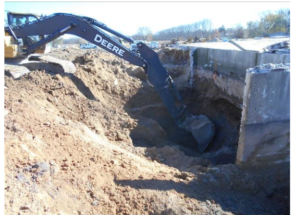
Photo #16 View looking east at east tank excavation after west tank removed. This is the "vault" for the soil excavated from soil boring B-7 area.
