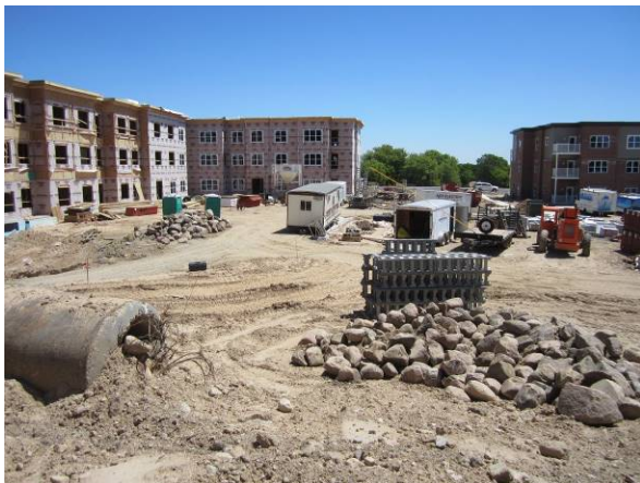
Photo #21 View looking east at redevelopment activities near north portion of site.
