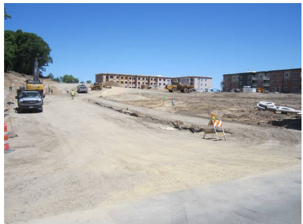
Photo #18 View looking north from south west corner of site after remedial activities completed and during redevelopment.
