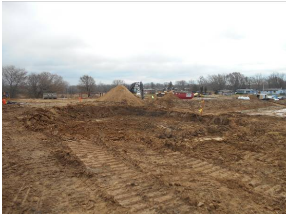
Photo #9 View looking east at B-10 excavation area after excavation was completed.
