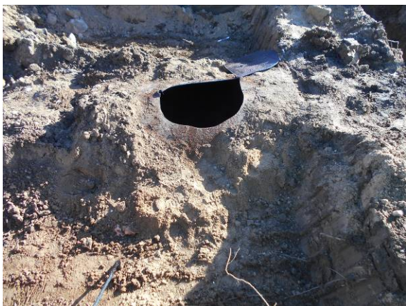
Photo #11 View of west tank prior to removal, after liquid removal and cleaning.
