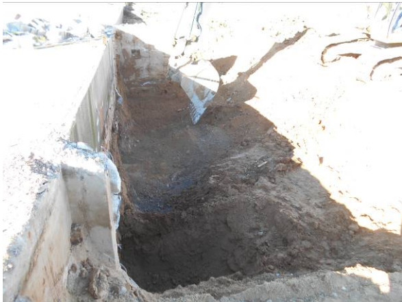
Photo #15 View looking west at east tank excavation after west tank removed.
