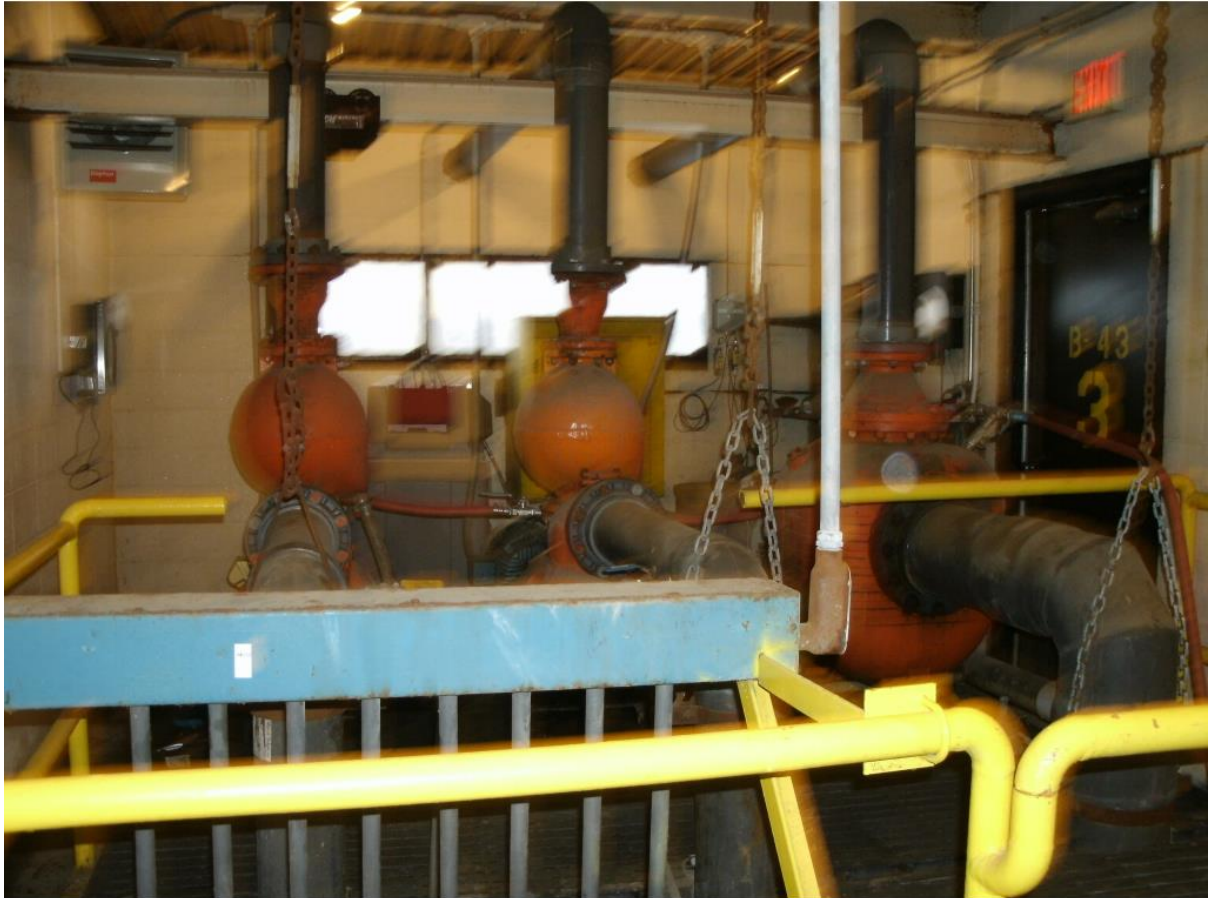
Pumps at Outfall 001
