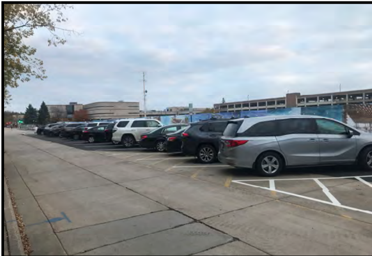
Asphalt cap currently used as angled parking along northern property boundary at Washington Street (11/01/2021)
