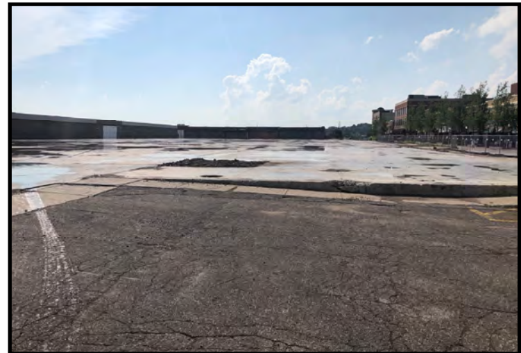
Concrete cap following rain event (09/16/2021)
