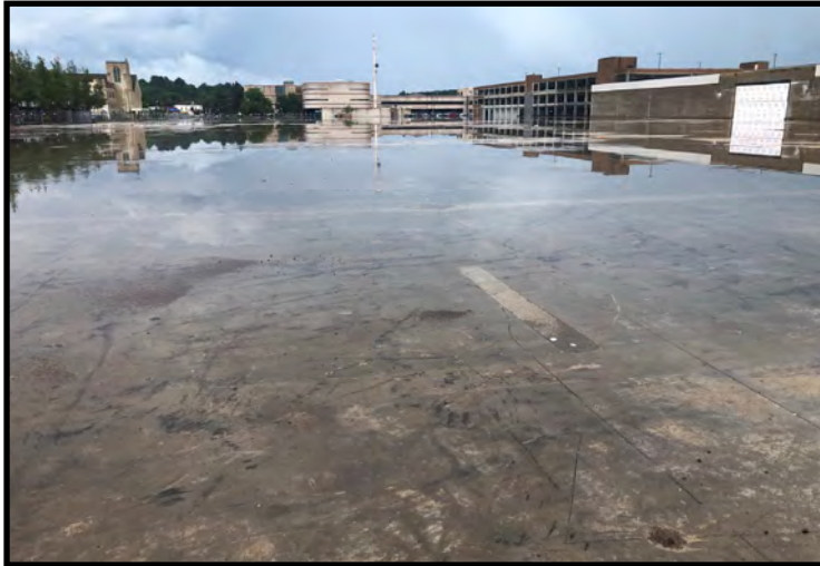
Concrete cap following rain event (09/16/2021)
