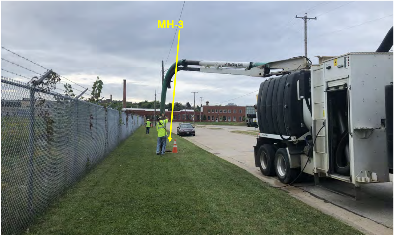
Photo 11: XPose (hydrovac contractor) conducting hydrovac excavation to the northeast of manhole MH-3. View to south; photograph taken on September 20, 2021.
