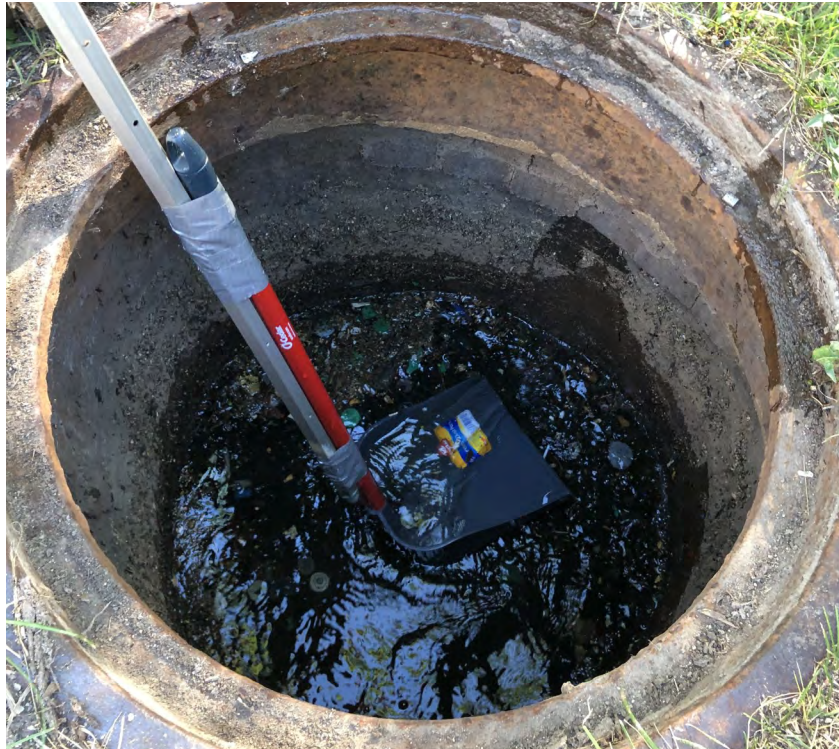
Photo 2: Manhole MH-1 interior with litter, debris, and grass. View to east; photograph taken on September 1, 2021.
