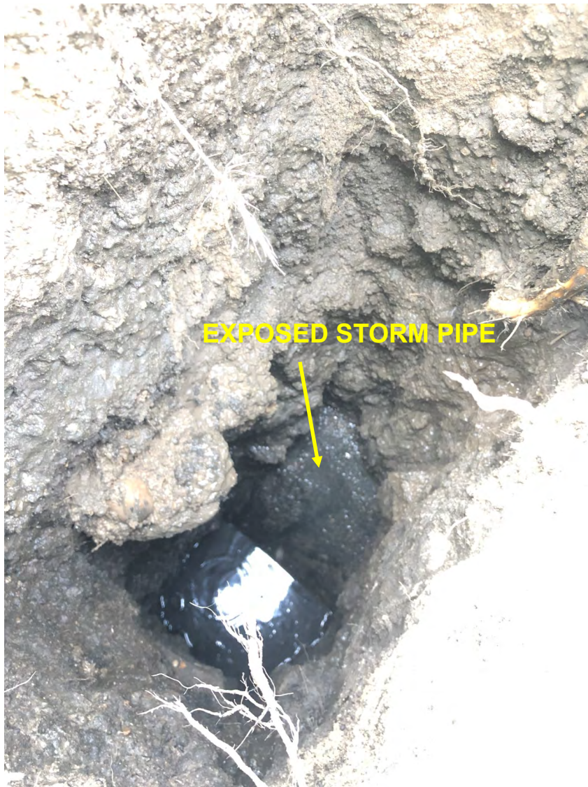
Photo 12: The open HydroVac excavation northeast of manhole MH-3. Exposed stormwater pipe. View to west; photograph taken on September 20, 2021.
