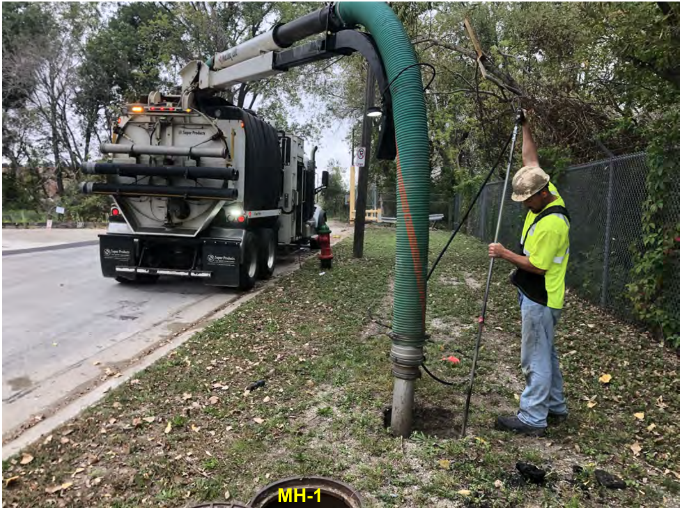
Photo 1: XPose (hydrovac contractor) conducting hydrovac excavation to the northeast of manhole MH-1. View to north; photograph taken on September 20, 2021.
