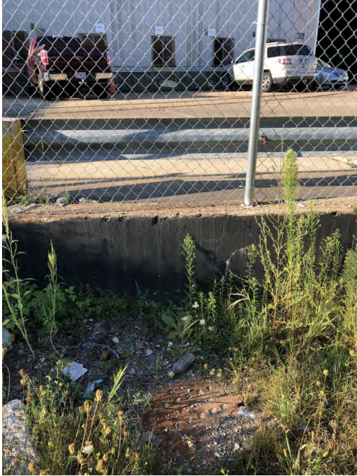
Photo 18: Manhole MH-15 exterior north of fence and elevated concrete-paved loading dock of 427 E. Stewart Street property. View to south; photograph taken on September 2, 2021.
