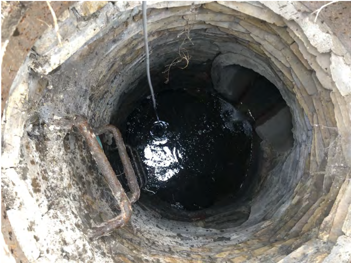
Photo 15: Manhole MH-5 interior with black, silty water. E Invert (on right). View to east; photograph taken on October 4, 2021.
