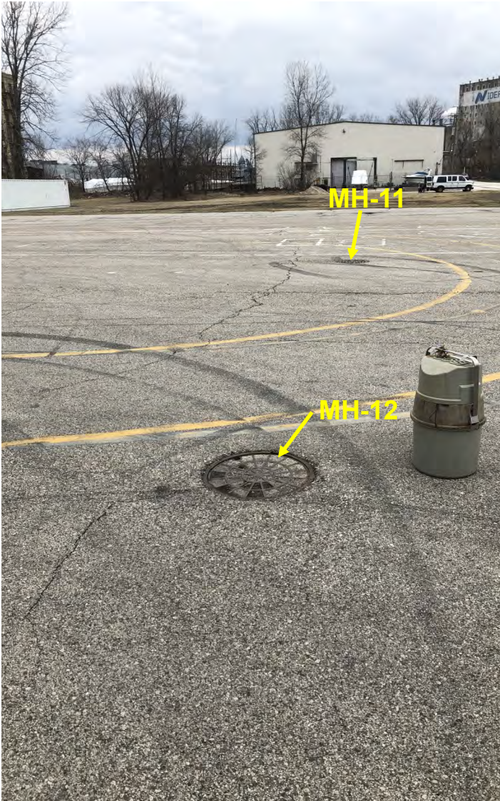
Photo 26: Manhole MH-12 exterior in 1982 S. Hilbert Street property parking lot, with manhole MH-11 in distance. View to north; photograph taken on April 4, 2022.
