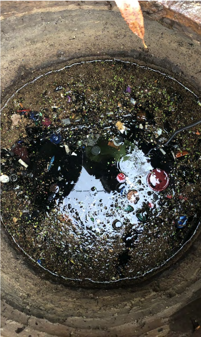
Photo 10: Manhole MH-1 interior with litter, debris, and grass. View to east; photograph taken on October 4, 2021.
