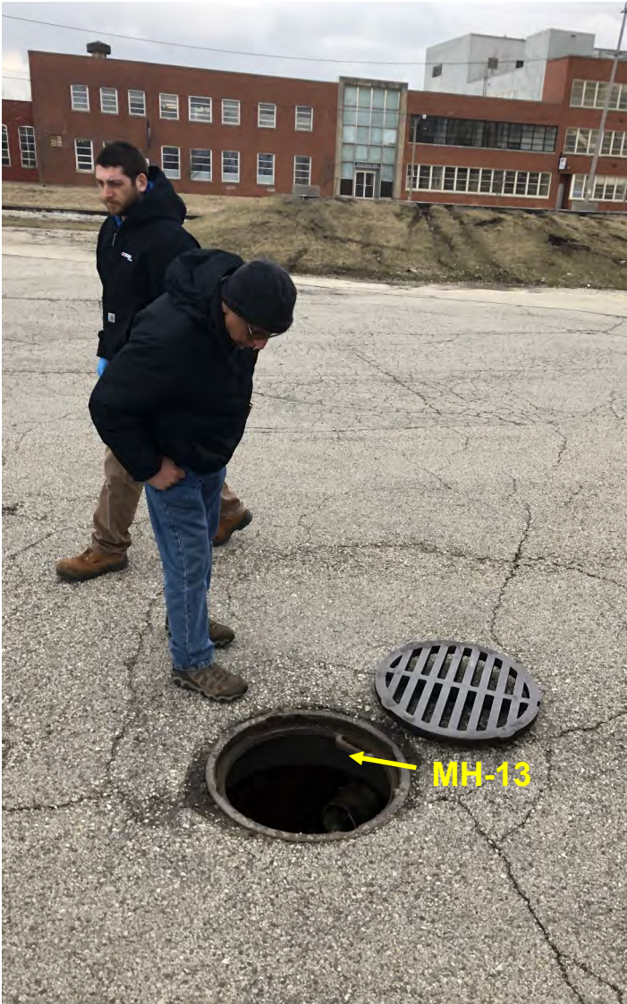
Photo 28: Manhole MH-13 exterior in 1982 S. Hilbert Street property parking lot. View to south; photograph taken on April 4, 2022.
