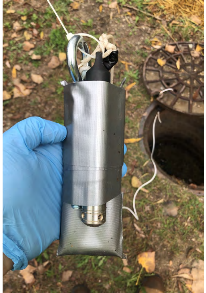
Photo 11: Levellogger MH-1 setup. Rope tied to manhole cover due to lack of ladder. View to northeast; photograph taken on October 4, 2021.
