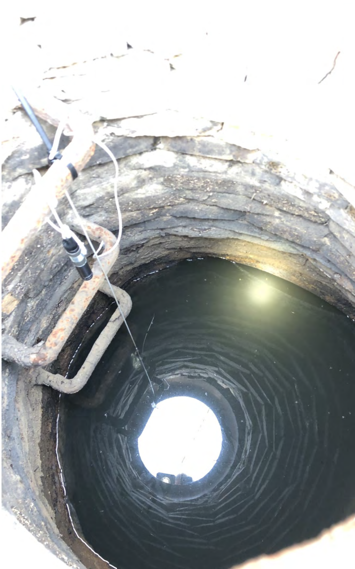
Photo 22: Manhole MH-4 interior with black silty water. View to northwest; photograph taken on October 11, 2021.
