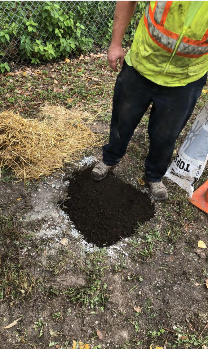
Photo 5: Geoprobe boring (MH-1-BF) borehole northeast of manhole MH-1 resurfaced with topsoil. View to southeast; photograph taken on September 20, 2021.
