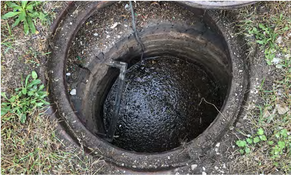
Photo 12: Manhole MH-2 interior with debris. View to north; photograph taken on October 4, 2021.
