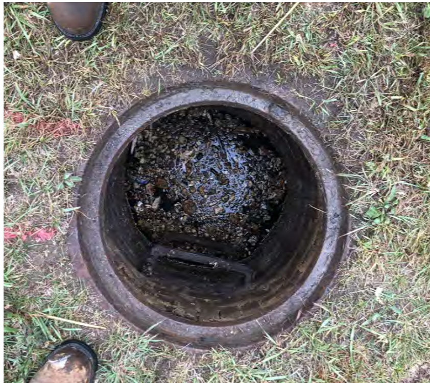
Photo 13: Manhole MH-3 interior with debris. View to east; photograph taken on October 4, 2021.
