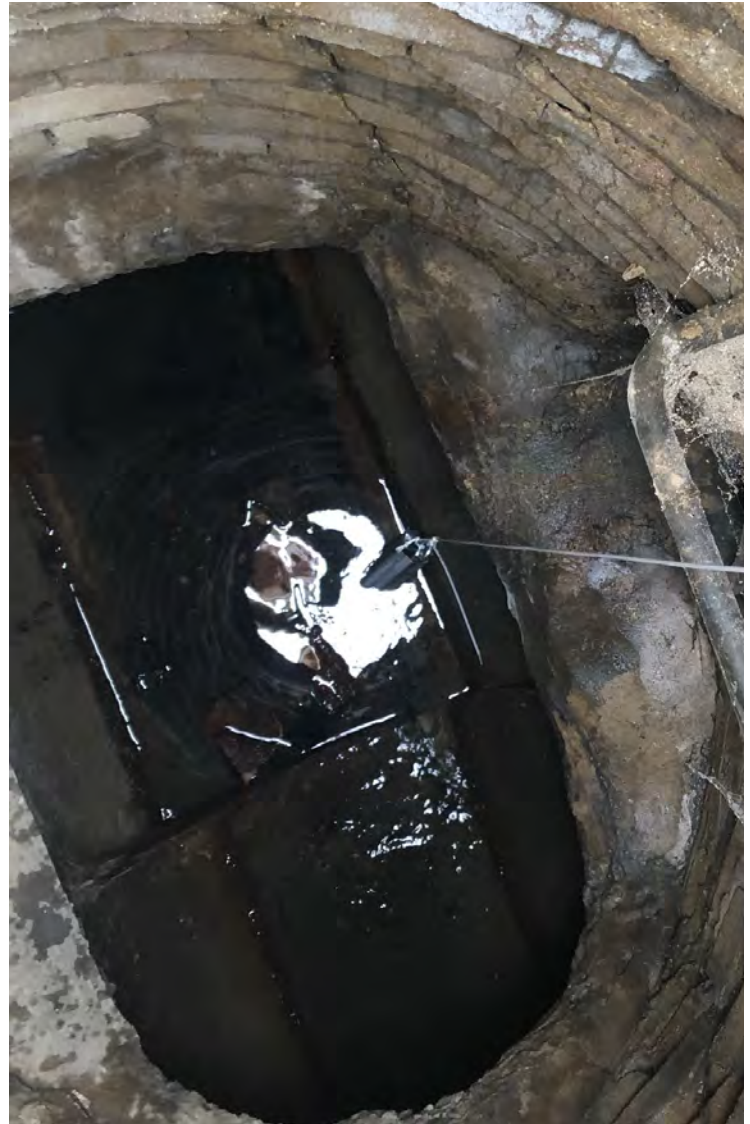
Photo 17: Manhole MH-14 interior, with trace sediment in the central portion of the pipe. Levellogger MH-14 tied to ladder on south side. View to southeast; photograph taken on October 4, 2021.
