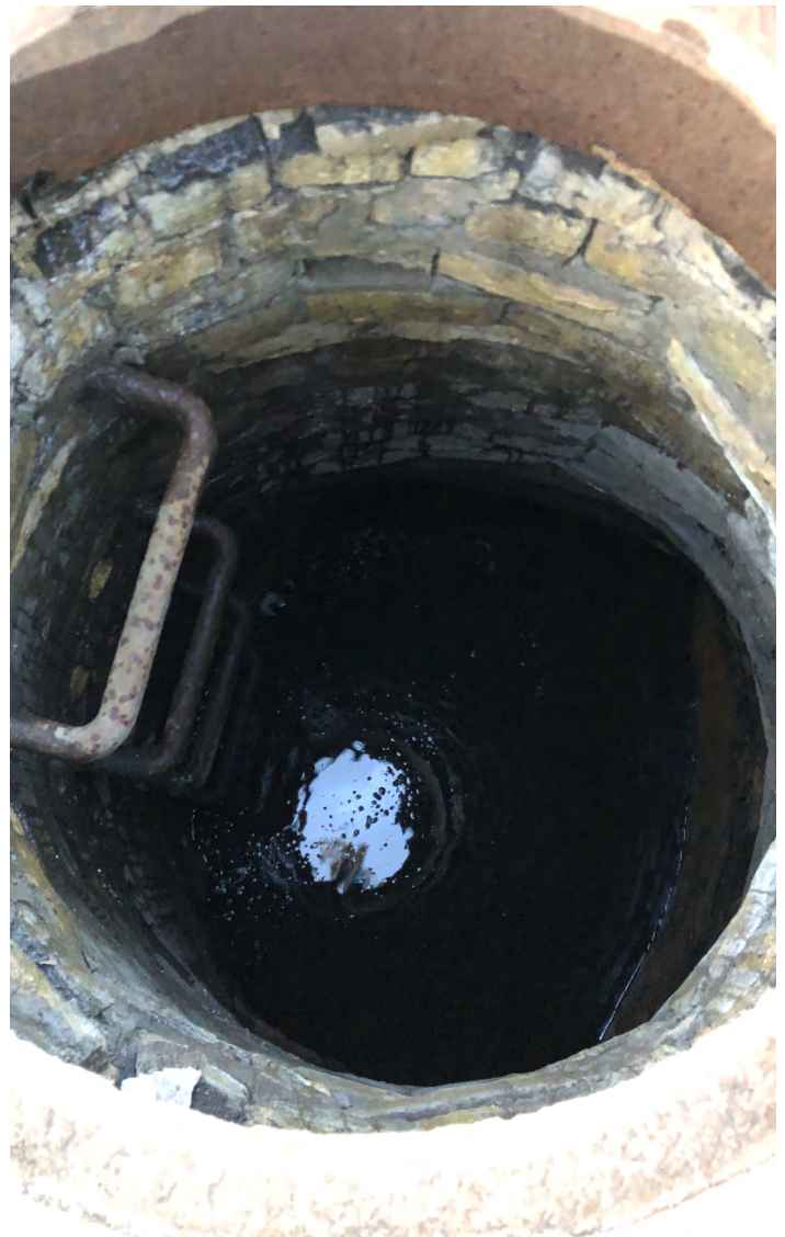
Photo 23: Manhole MH-4 interior with black silty water. View to northwest; photograph taken on February 28, 2022.
