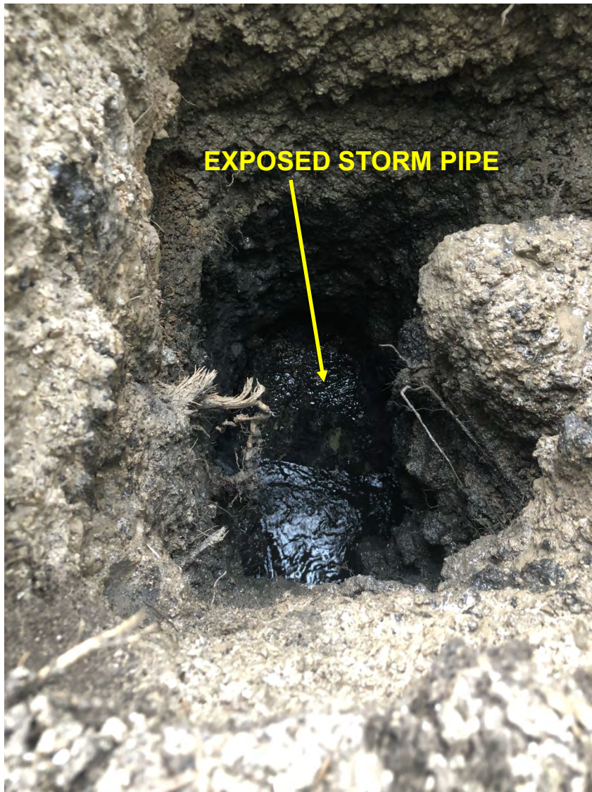
Photo 2: The open HydroVac excavation northeast of manhole MH-1. View to west; photograph taken on September 20, 2021.
