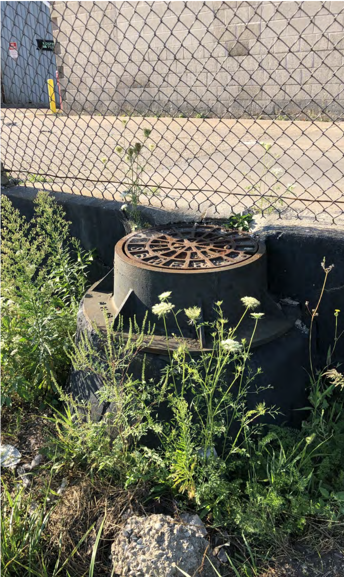
Photo 16: Manhole MH-14 elevated approximately 2.6 feet above neighboring ground surface. View to south; photograph taken on September 2, 2021.
