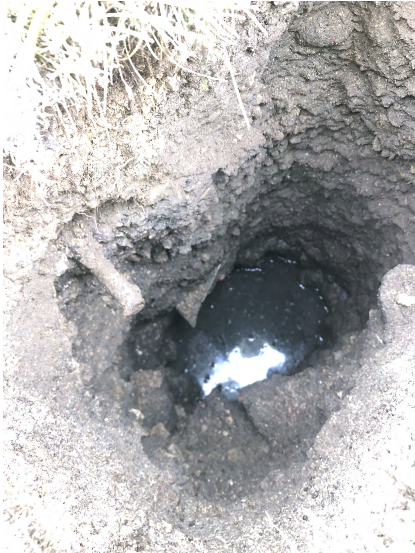
Photo 8: The open HydroVac excavation northeast of manhole MH-2. Water recharged rapidly to cover pipe. View to west; photograph taken on September 20, 2021.
