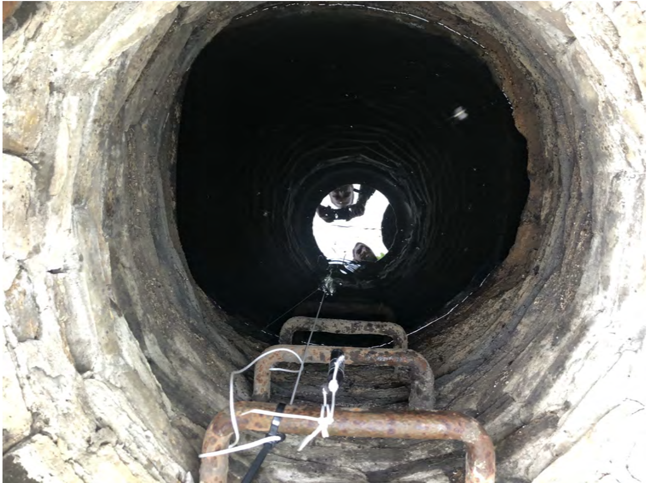
Photo 14: Manhole MH-4 interior with black silty water. Level logger for manhole MH-4 and barometric pressure logger tied to manhole ladder. View to east; photograph taken on October 4, 2021.
