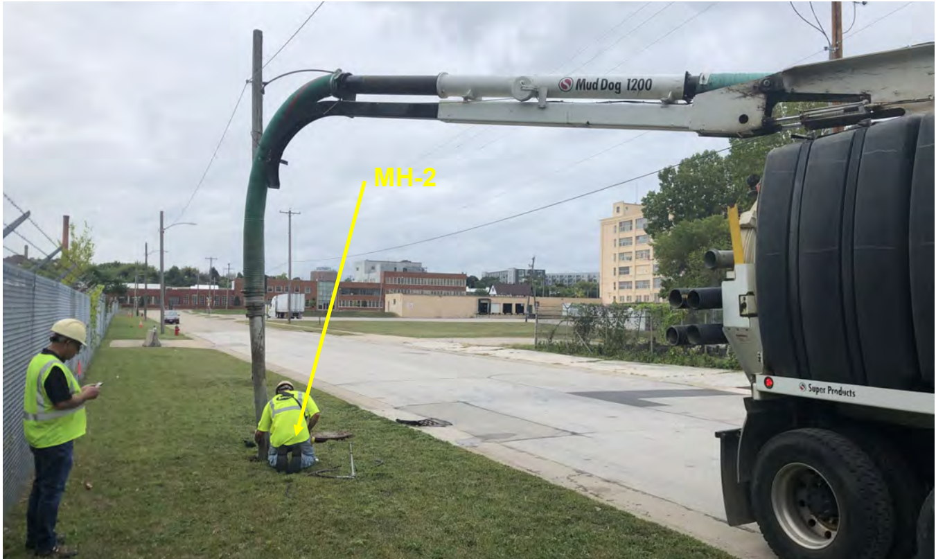
Photo 7: XPose (hydrovac contractor) conducting hydrovac excavation to the northeast of manhole MH-2. View to southwest; photograph taken on September 20, 2021.
