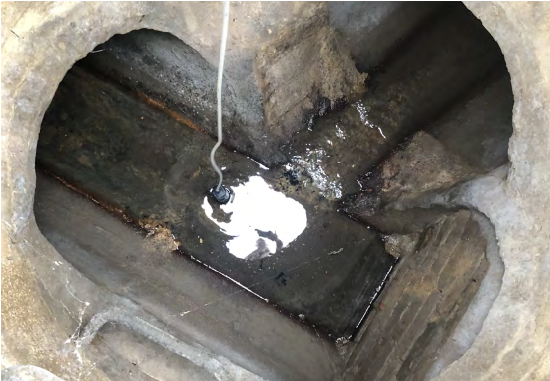
Photo 19: Manhole MH-15 interior with trace sediment and low water column. S invert (left) and W invert (right). View to southwest; photograph taken on October 4, 2021.
