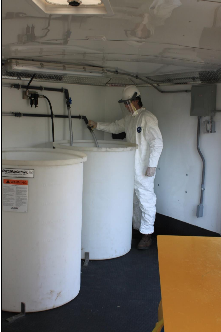
Figure 3 Enclosed chemical mixing system.
