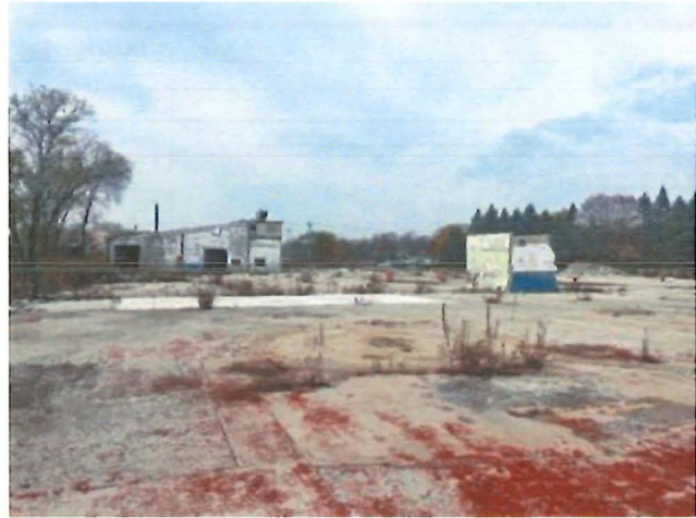
IMAGE 2: VIEW SOUTHEAST OF AMCAST NORTH, SHOWING THE PARTIALLY DEMOLISHED BUILDING, OLD UNDERGROUND PARKING ACCESS, AND PAVED AREAS.
