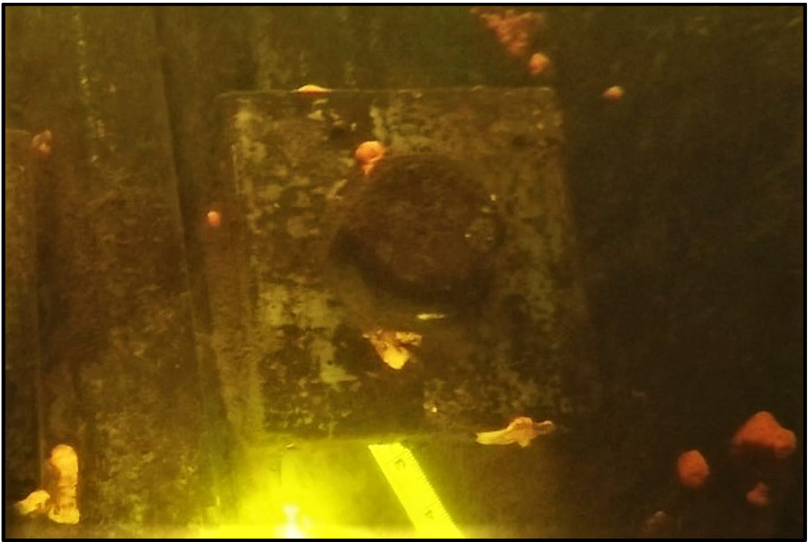
PHOTO 6. Underwater view of a ruler penetrating 2.75 inches into the gap between the washer plate and steel sheet pile.
