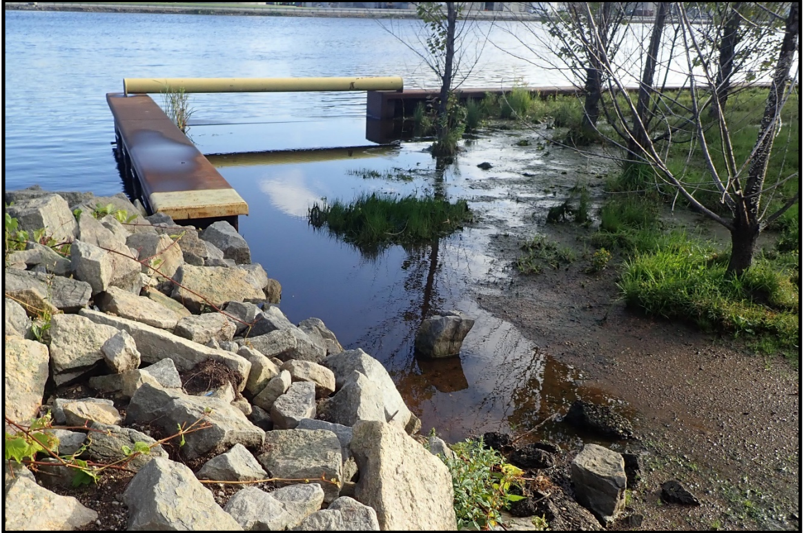
PHOTO 13. View of localized erosion at the weir at the western extent of the structure, looking north.
