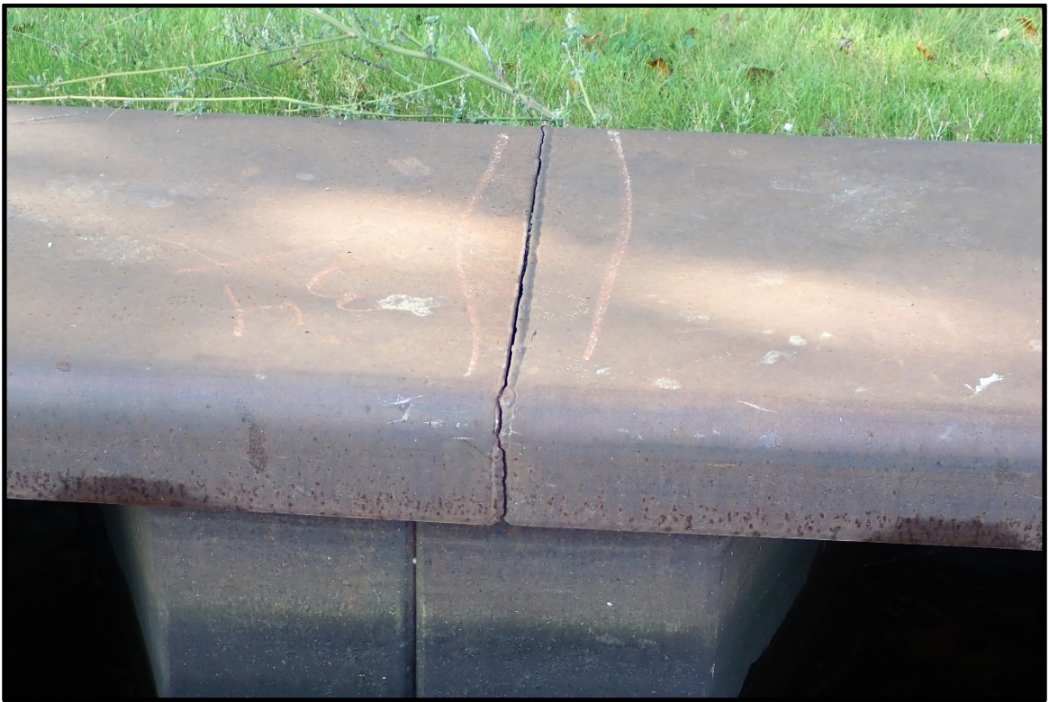
PHOTO 10. View of the cracked weld in the steel bent plate cap at approximately 12 ft past D-6, looking south.
