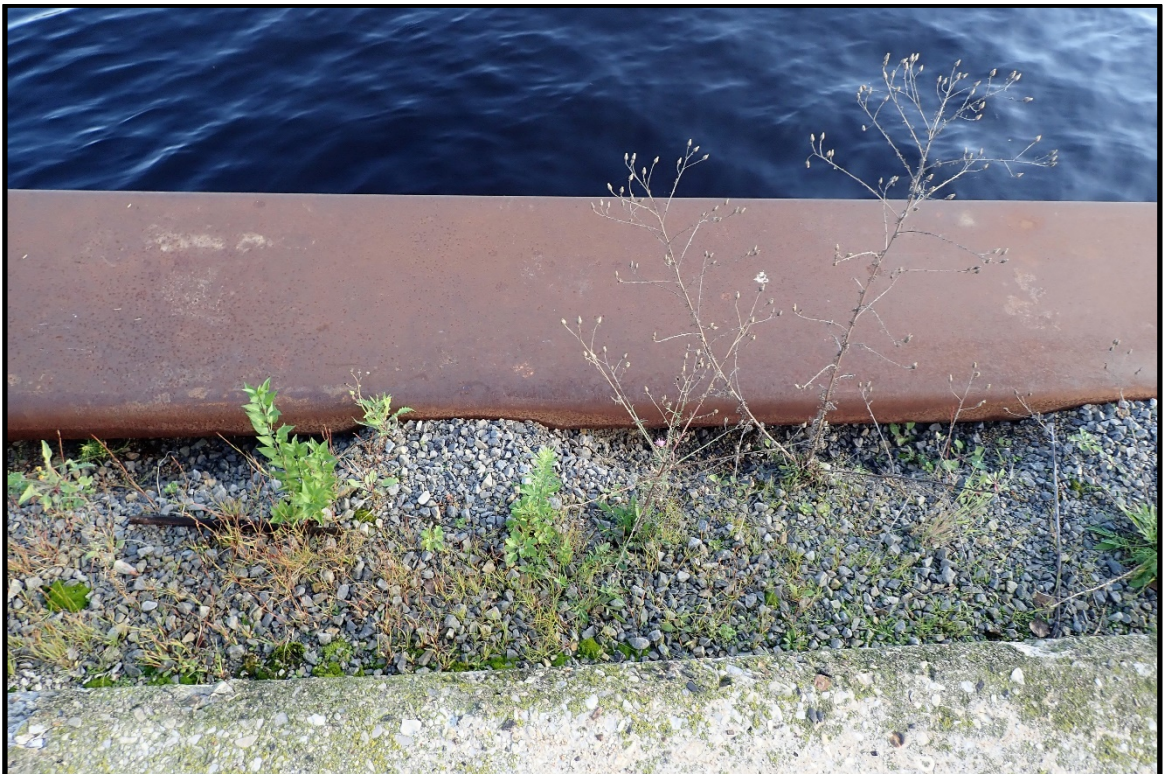
PHOTO 12. View of typical localized erosion on the land side of the barrier wall, looking north.
