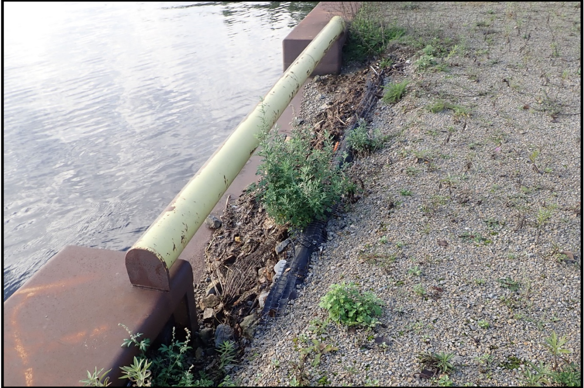
PHOTO 5. View of a typical weir cut in the barrier wall at approximately 10 ft past D-23, looking south.
