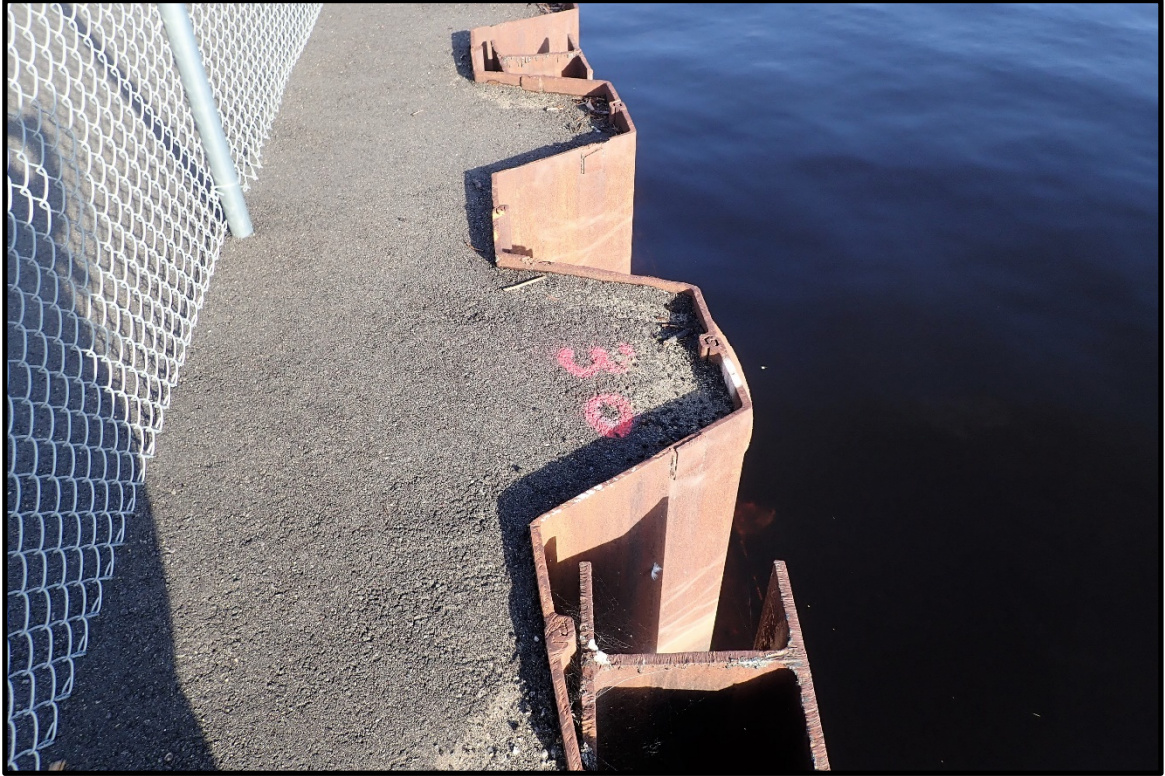
PHOTO 3. View of barrier wall at Dimple Point D-30 with offshore H-piles, looking northwest.
