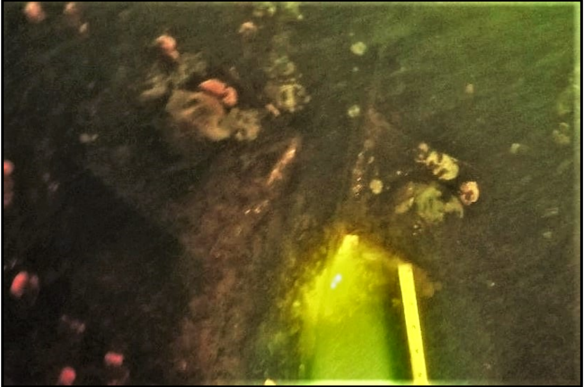
PHOTO 7. Underwater view of the broken washer plate at approximately 35 ft past D-12, looking south.
