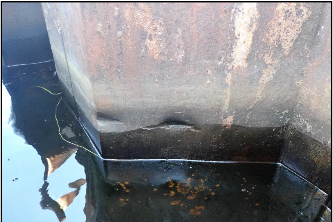
PHOTO 8. View of minor impact damage on the steel sheet pile at approximately 42 ft past D-30, looking southeast.
