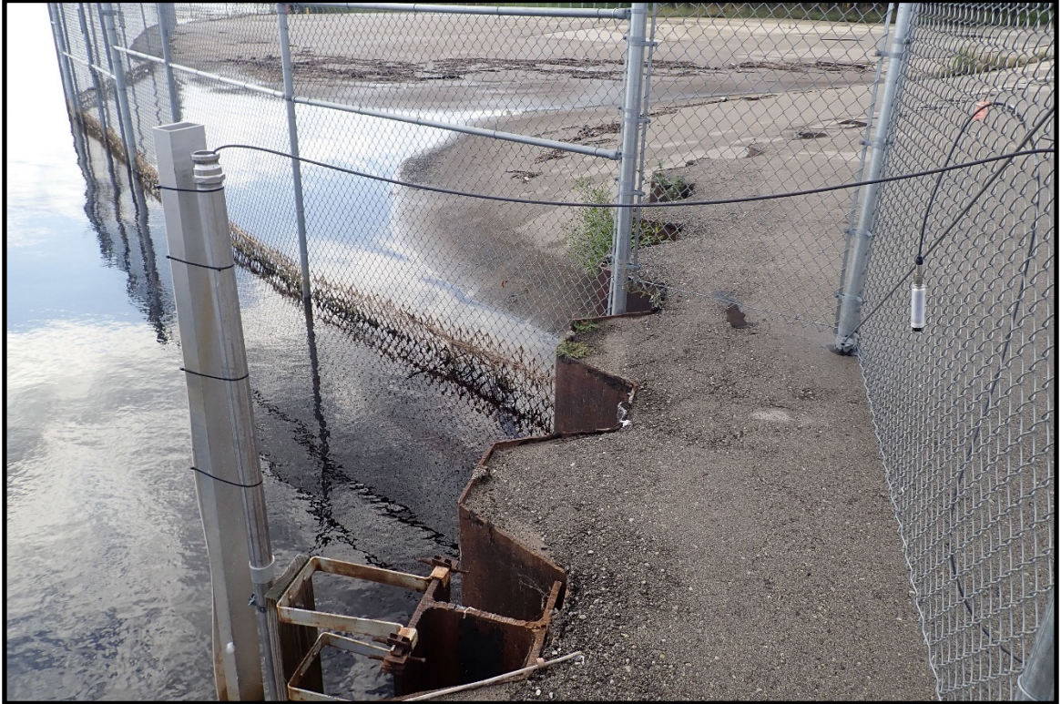
PHOTO 9. Above water view of the transition between generations of VBW at PT “F”, looking south. The chain link fence follows the submerged 2010 barrier wall.
