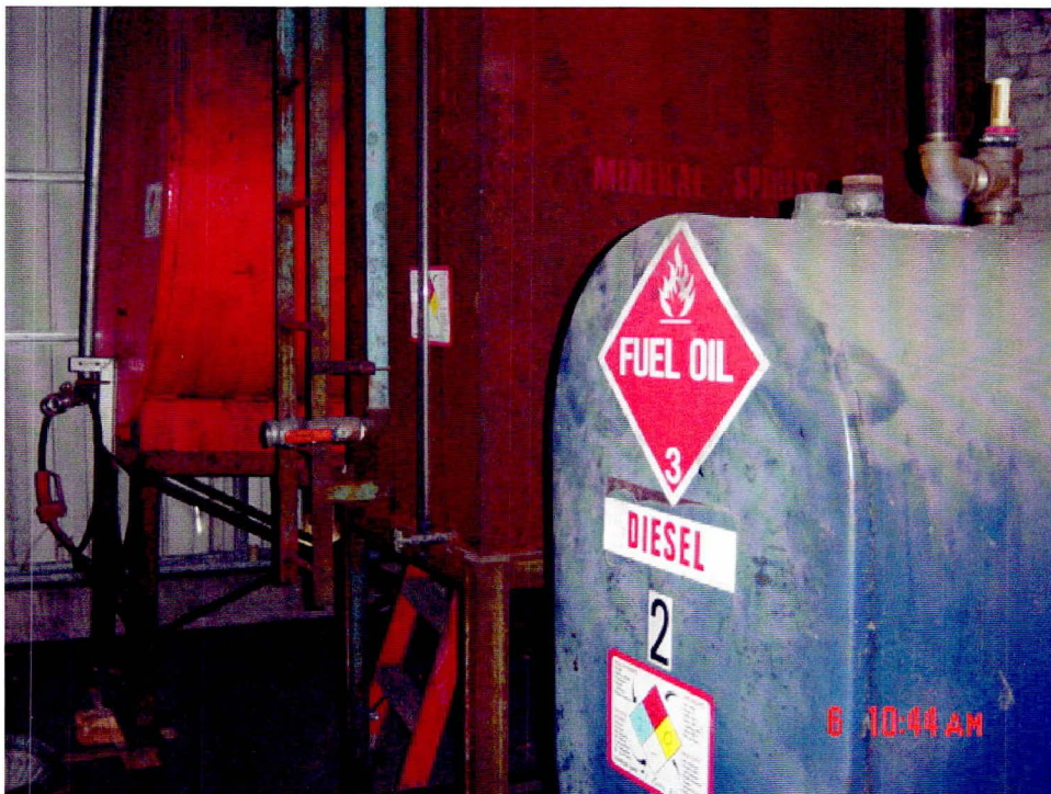
Three ASTs in Building 13.
