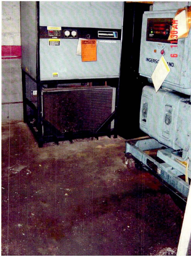
Staining on concrete floor, adjacent to compressors in Building 22.
