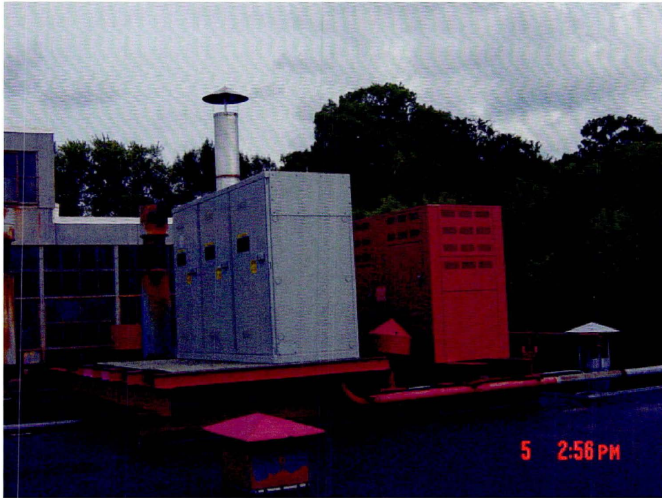
Transformers located on top of Building 5.
