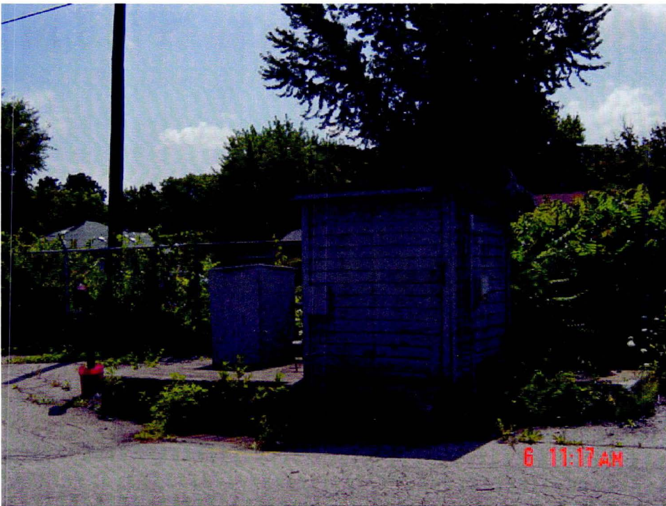
Sewer lift station, southeastern property corner.
