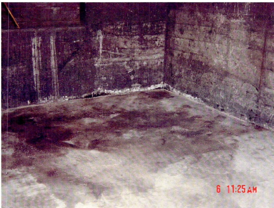
Stained floor, hazardous waste accumulation area, Building 23B.
