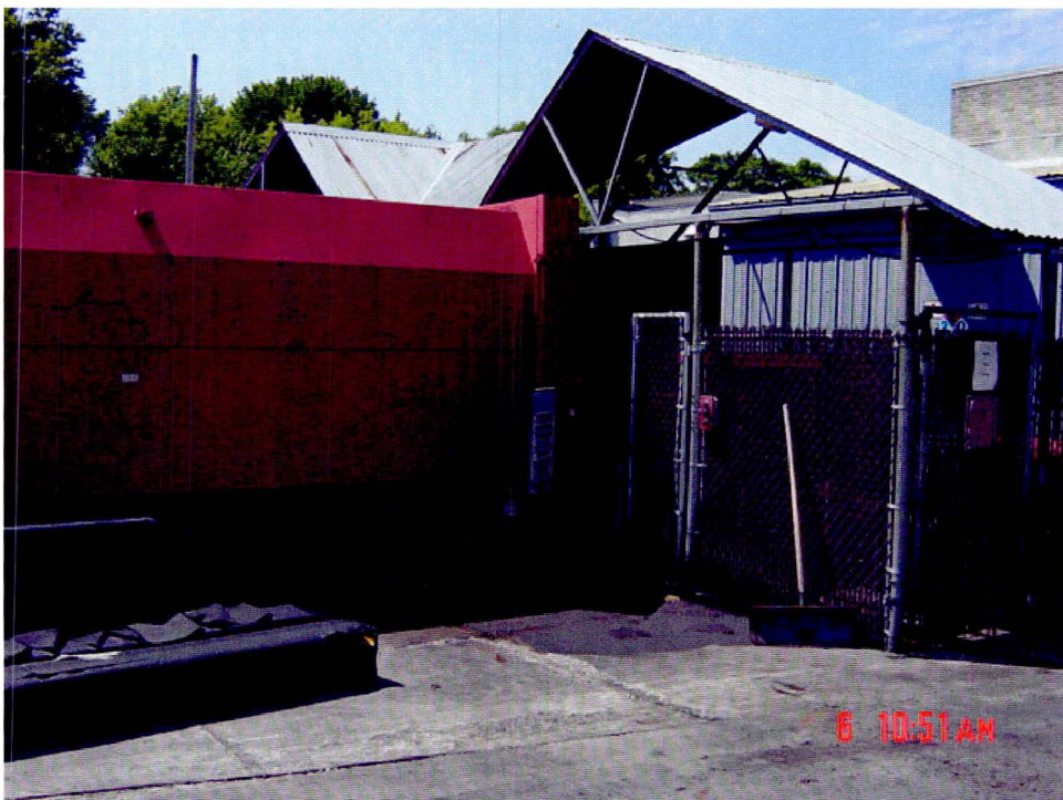
Stained concrete adjacent to two trash compactors, eastern side of Building 2.
