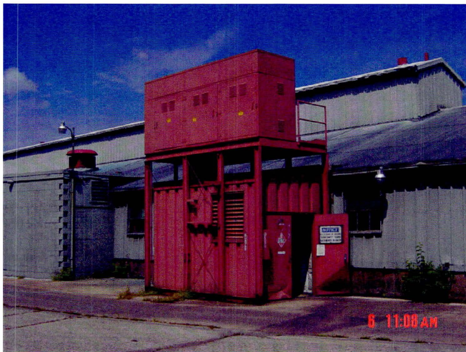
Transformer located on building adjacent to the southern side of Building 12C.
