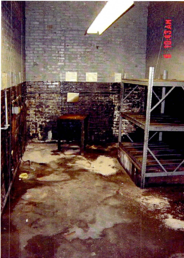
Stained concrete floor, flammable storage room, Building 16.
