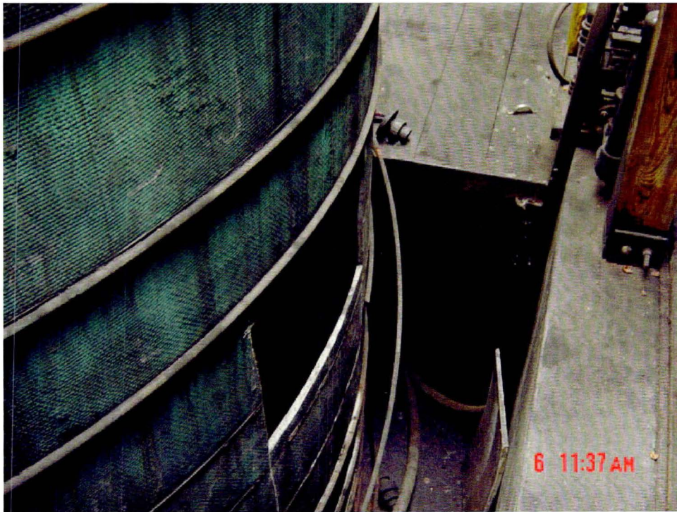
Hole placed in zinc chloride AST, Building 7.
