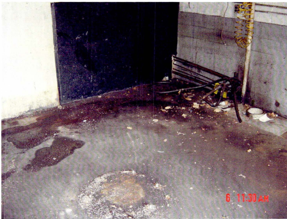
Staining on concrete floor, Building 22.
