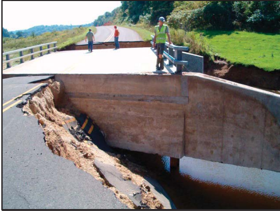
Figure 11: Bridge in Vernon County compromised by the August, 2007 flood.
