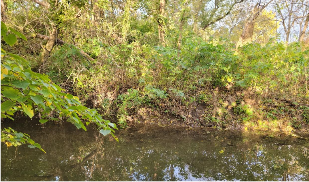
Severe undercut with vegetative overhang and exposed tree roots.
