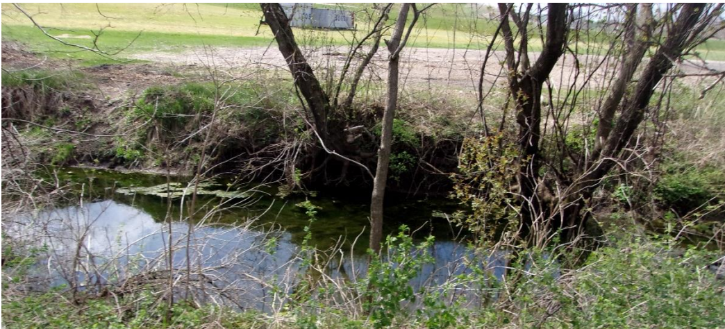
Severe undercut with slump, vegetative overhang, and exposed tree roots.
