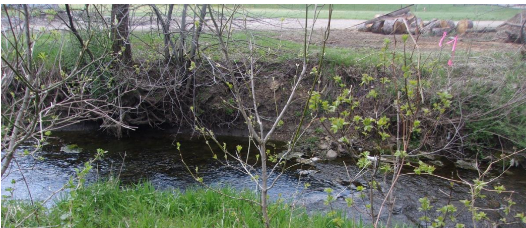
Severe undercut with slump, vegetative overhang, and exposed tree roots.
