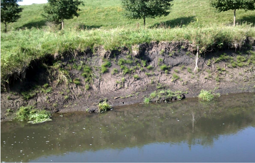
Image 12 – Bare bank, severe undercut with slump and vegetative overhang.
