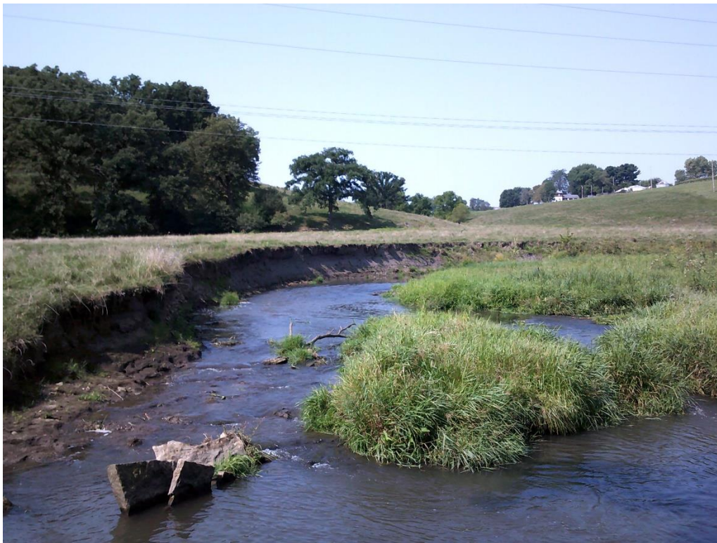
Image 5 – Bare bank, severe undercut with slump and vegetative overhang.
