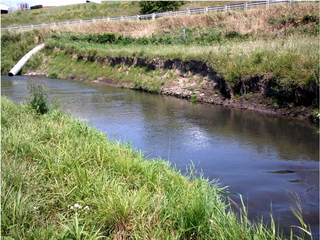
Image 9 – Bare bank, severe undercut with slump, exposed culvert, and vegetative overhang.
