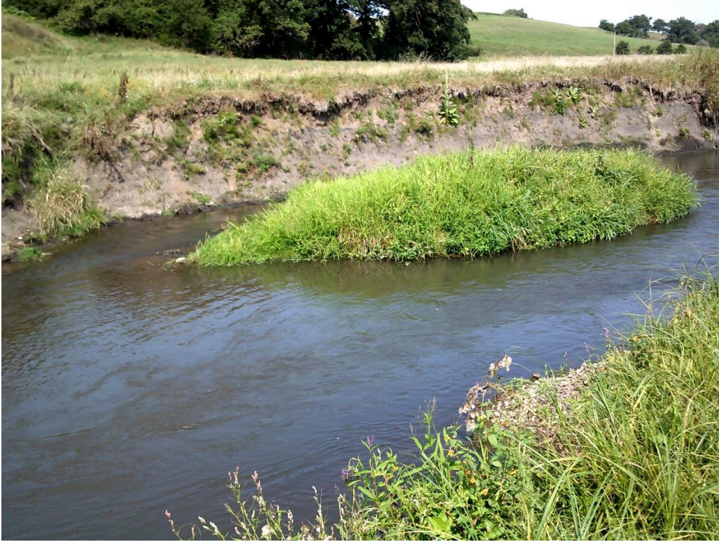
Image 2 – Bare bank and severe undercut with slump.
