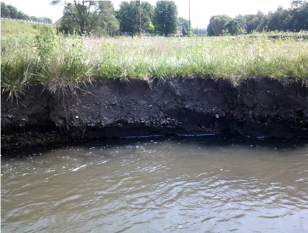
Image 3 – Bare bank, severe undercut and vegetative overhang.
