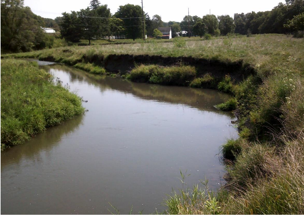
Image 10 – Bare bank, severe undercut with slump and vegetative overhang.
