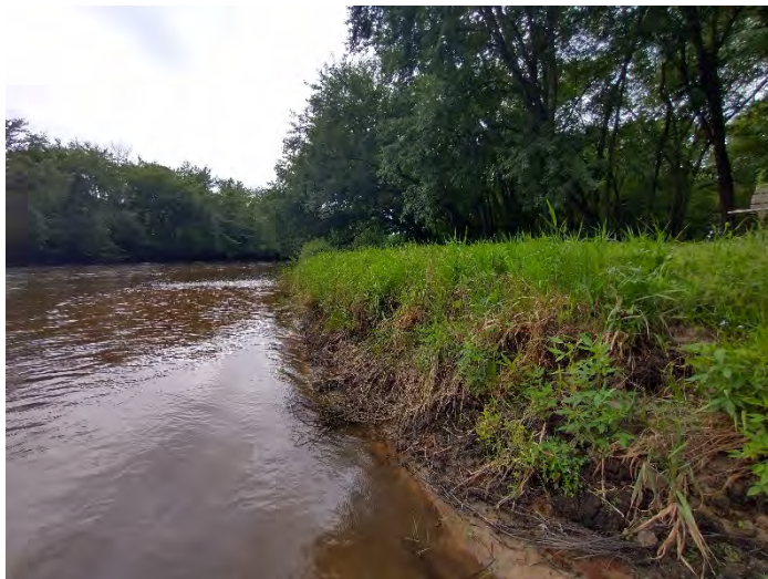
7: Vertical banks and erosion, north bank
