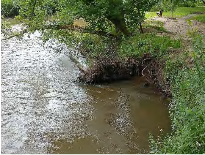
1: Scour hole in north bank of river
