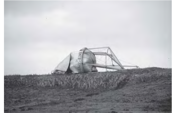
A water tower that has exceeded its useful life!
