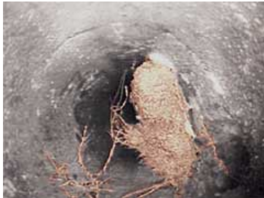
Roots growing into a sewer collection pipe
