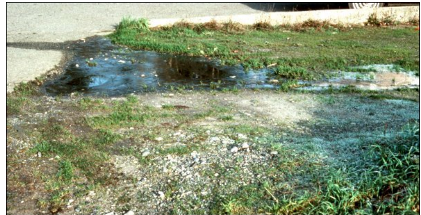
Failed leaching trench results in surface breakout
