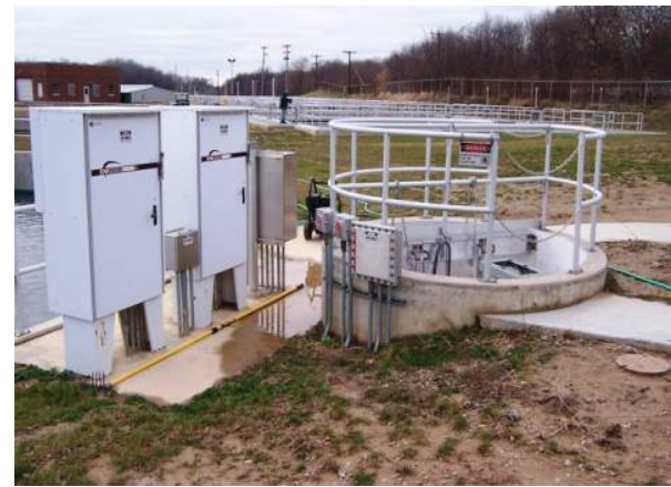
Return Activated Sludge (RAS) station and two associated Pad Mounted Transformers (PMTs) Credit: City of Lincoln, IL
