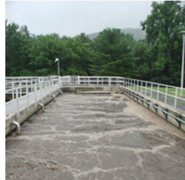
Aeration tank at a small wastewater facility
