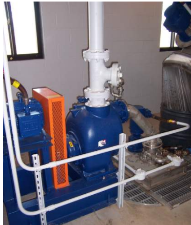
Grit removal and grinder/screener units Credit: Village of Boyd, WI
