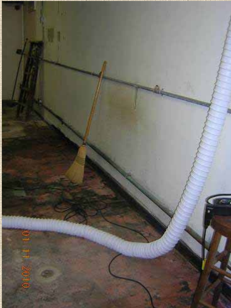
East wall – floor stained – GP3 in bottom left corner (1,900 ug/kg PCE)
