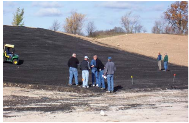
Kiel site following primary grading and distribution of PMR-foundry sand mix, October 2005.
