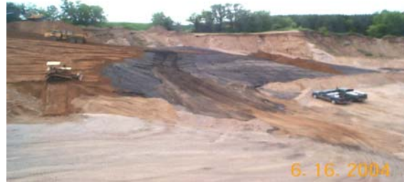
Foundry sand being incorporated as part of grading activities during reclamation of the Foley Pit (Photo by Dave Misterek, DNR)
