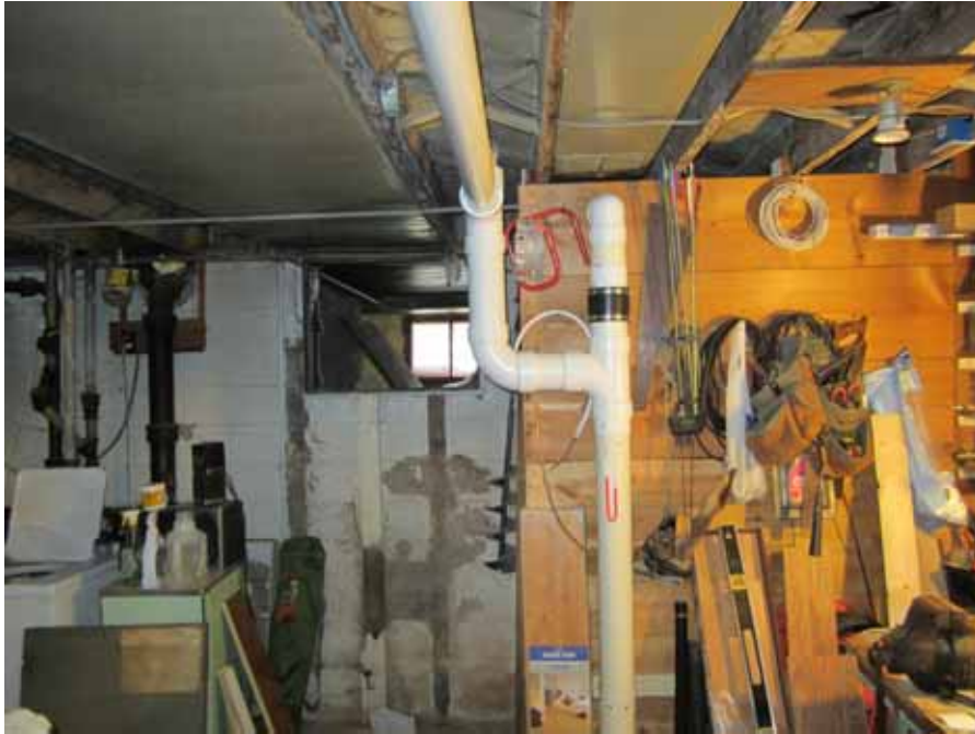
Basement Suction Piping
