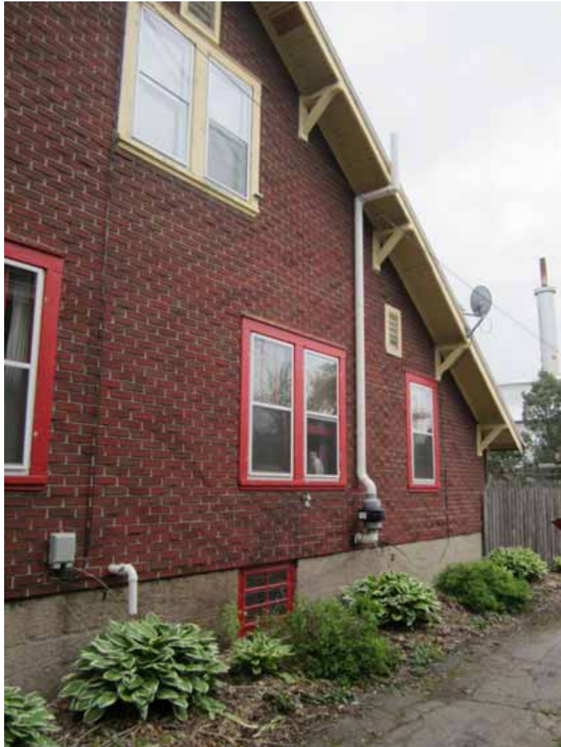
SSDS fan and discharge piping
