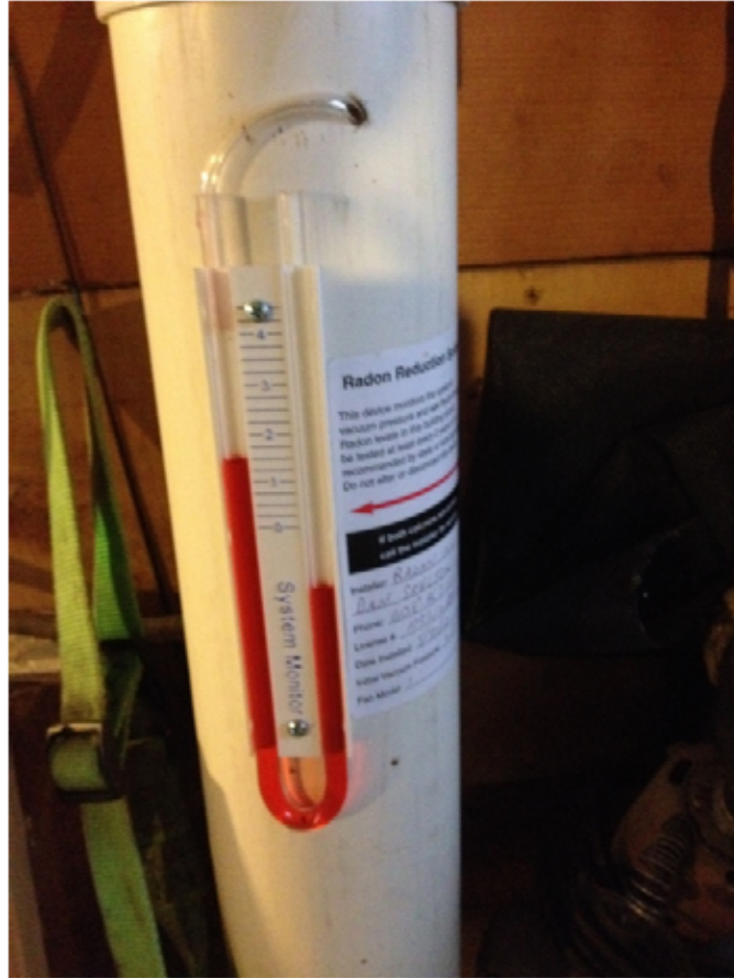
Manometer, operating level 1.50 in wc
