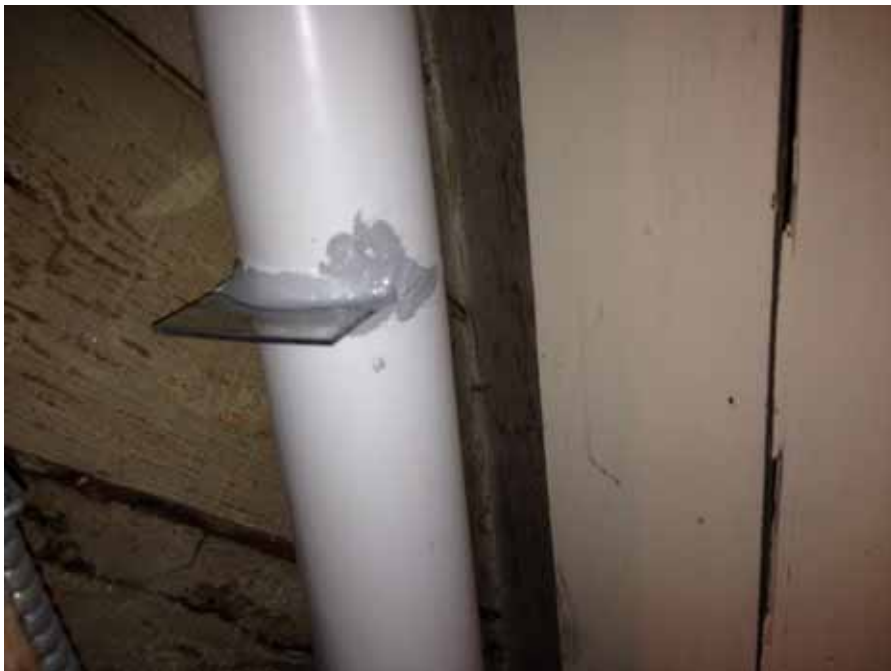
Damper in Piping to Crawlspace
