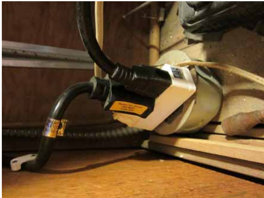
Labeled plug controlling SSDS fan
