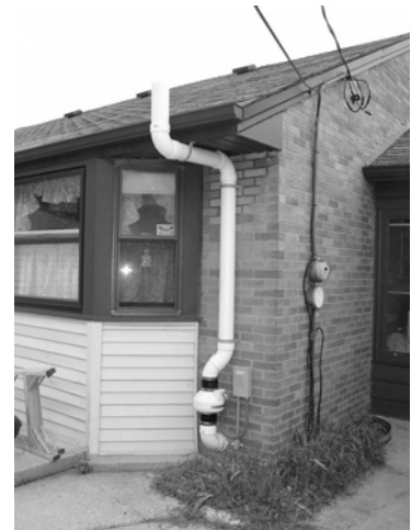
An example of a vapor mitigation system (courtesy: WI Department of Health)
