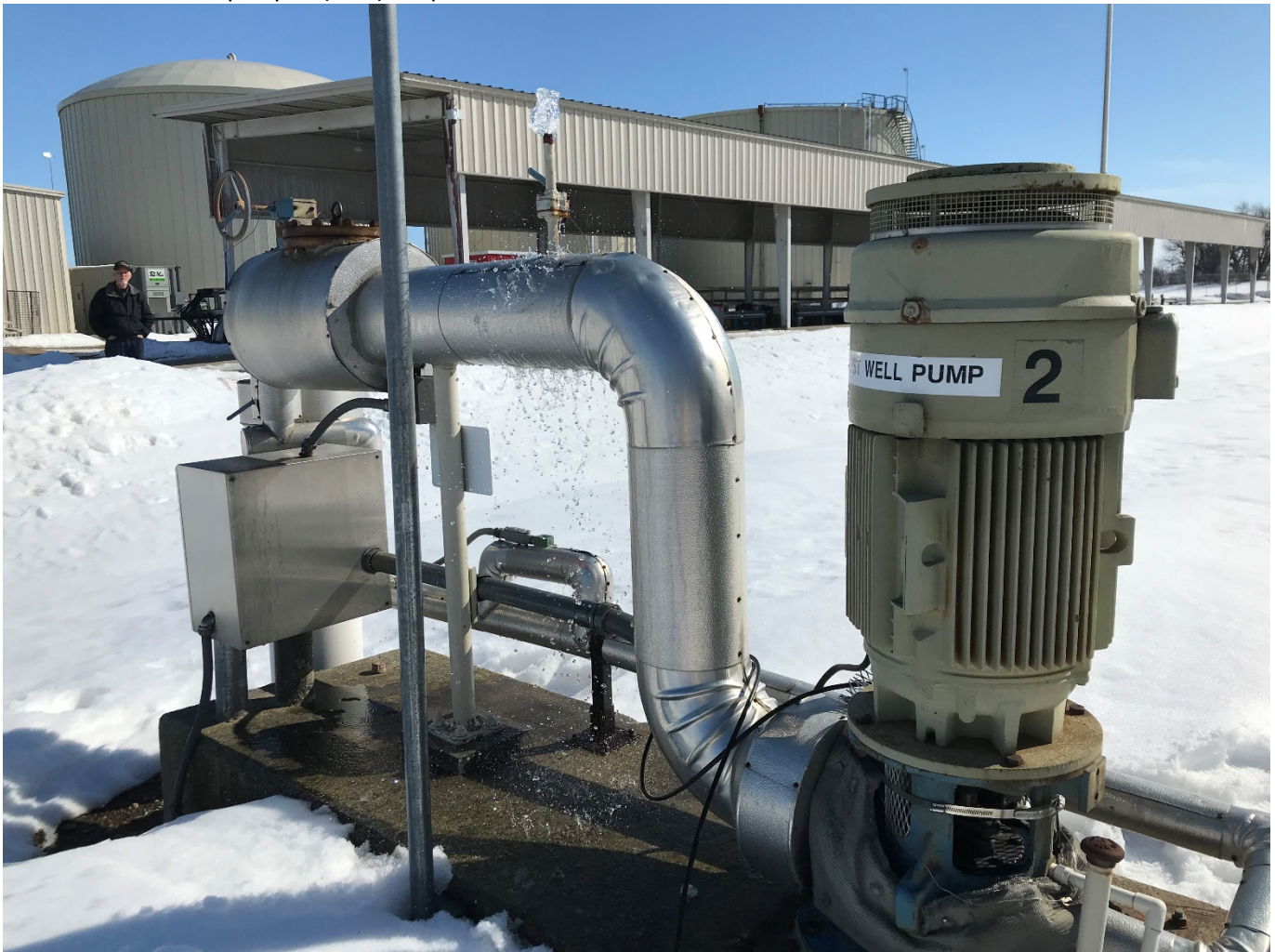
Production well water pump #2 (west) sample location
