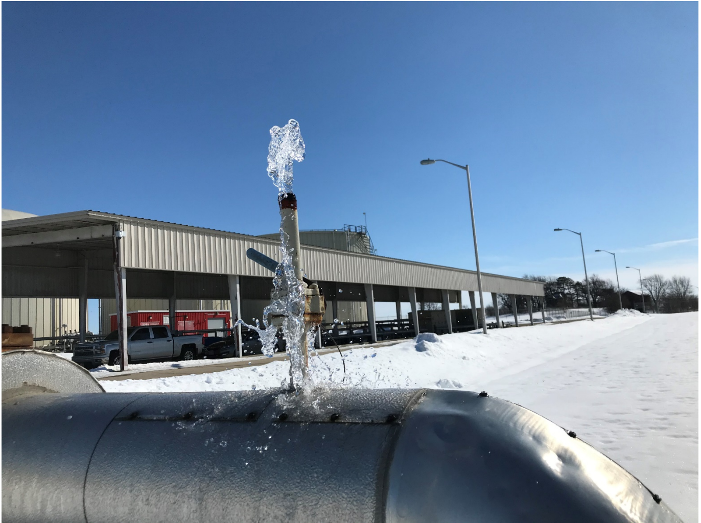
Production well water pump #2 (west) sample location close-up
