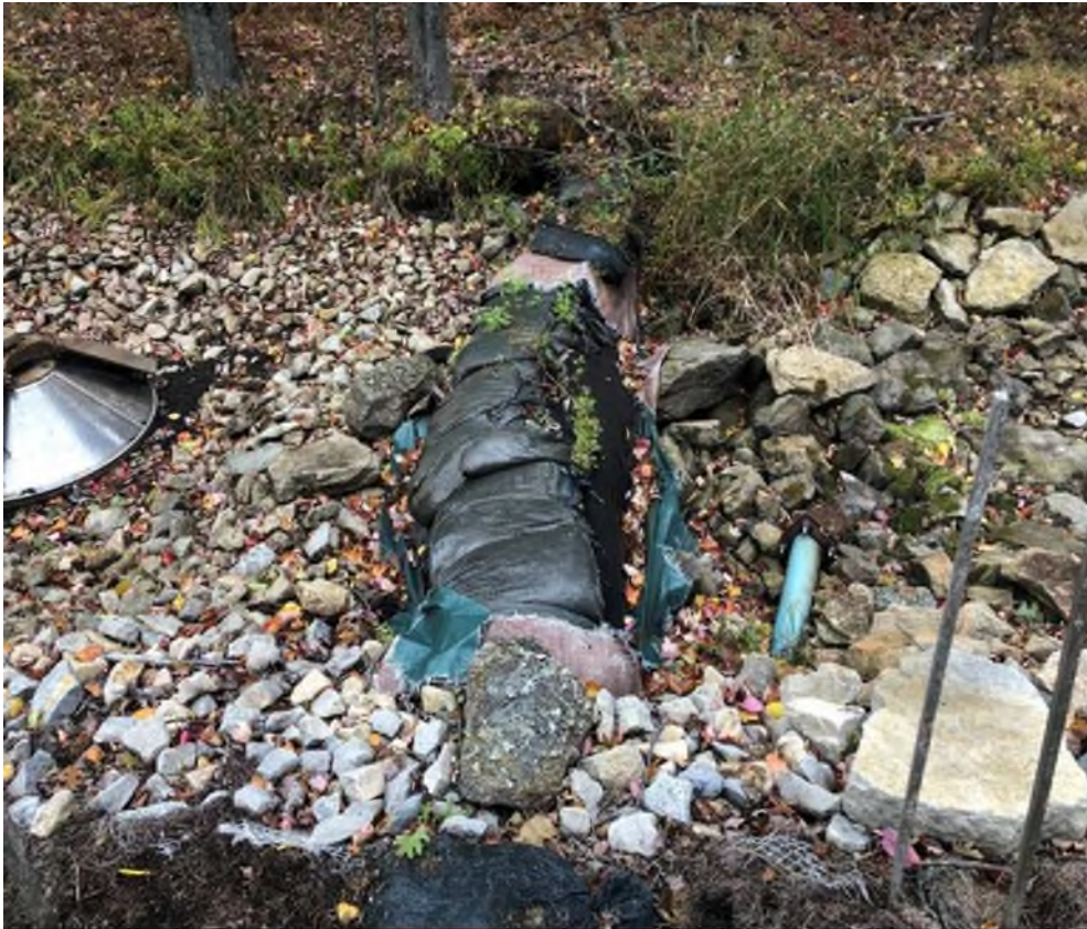
Photograph 1. Ditch A In-stream check dam condition prior to maintenance.
