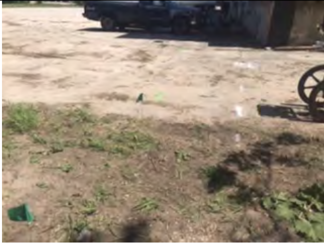
Outfall and unknown pipe
