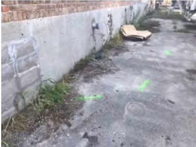
Outfall traced back to building
