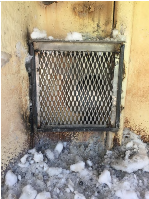
Photograph #15 Ashland/NSP Lakefront Site B14-02346.02 Date: April 29, 2020 BRAUN INTERTEC Subject: Typical cover for drain tile penetrations through the sheet pile wall
