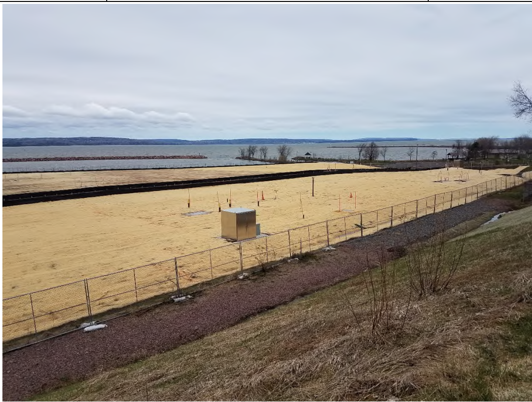
Photograph #16 Ashland/NSP Lakefront Site B14-02346.02 Date: April 29, 2020 BRAUN INTERTEC Subject: Erosion control blanket installed in Phases 3 and 4
