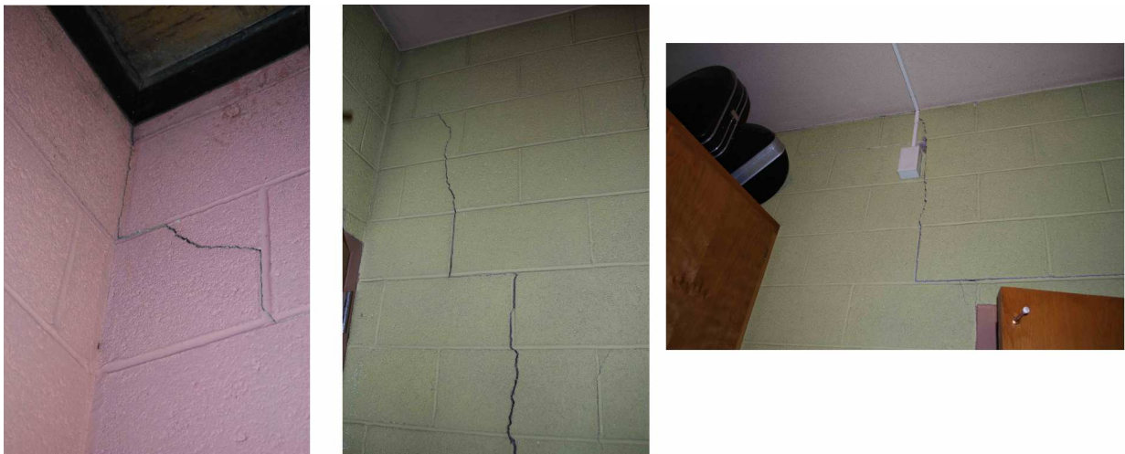
Figure 7- Existing cracks in the church to be monitored with crack gages
