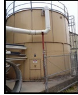
Non-pressure storage tanks (aka water storage facilities)
