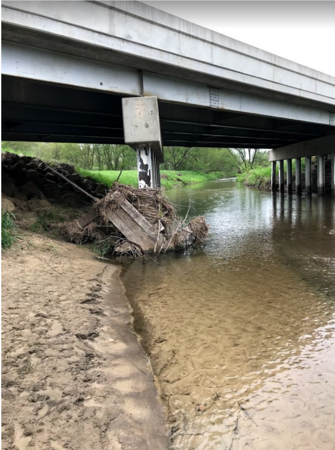
Figure 21. Failed LUNKER structure pinned against the HWY 82 Bridge over Otter Creek. Photo: Kirk Olson.
