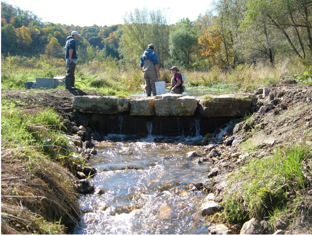
Fig. 6. Intentional trout passage barrier installed on Tenny Springs Creek in 2007. This structure was determined to be a partial barrier to Brown Trout, which re-colonized the reach in the years following installation and Brown Trout removal. Photo Credit: Matt Mitro.
